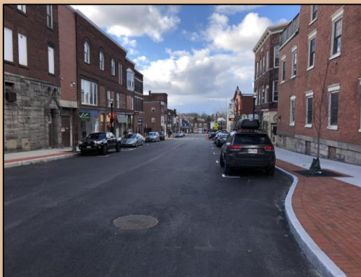
Reconstruction of Kingman Street Photo provided by the City of St. Albans
