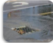
Photo: Road stormwater collection
