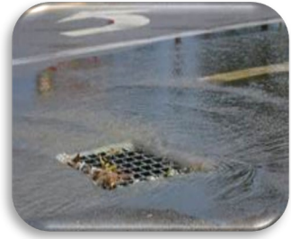
Photo: Road stormwater collection
