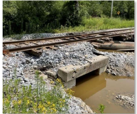
FIGURE 26 STORM DAMAGED RAIL LINES
