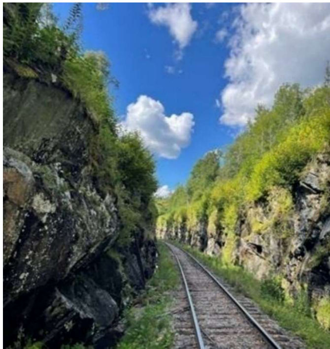
There are a variety of risks to operating rail service in Vermont. The GMRR between Bellows Falls and Rutland traverses rock cuts subject to rockfall, slope failure, and flooding.
