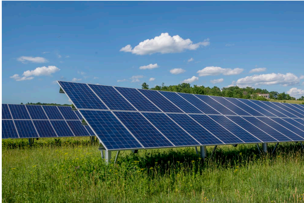
Solar Array in Ferrisburgh, VT
