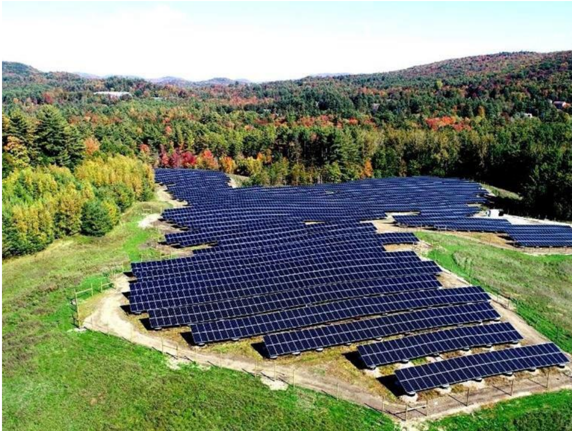
Photo courtesy of Encore Renewable Energy
