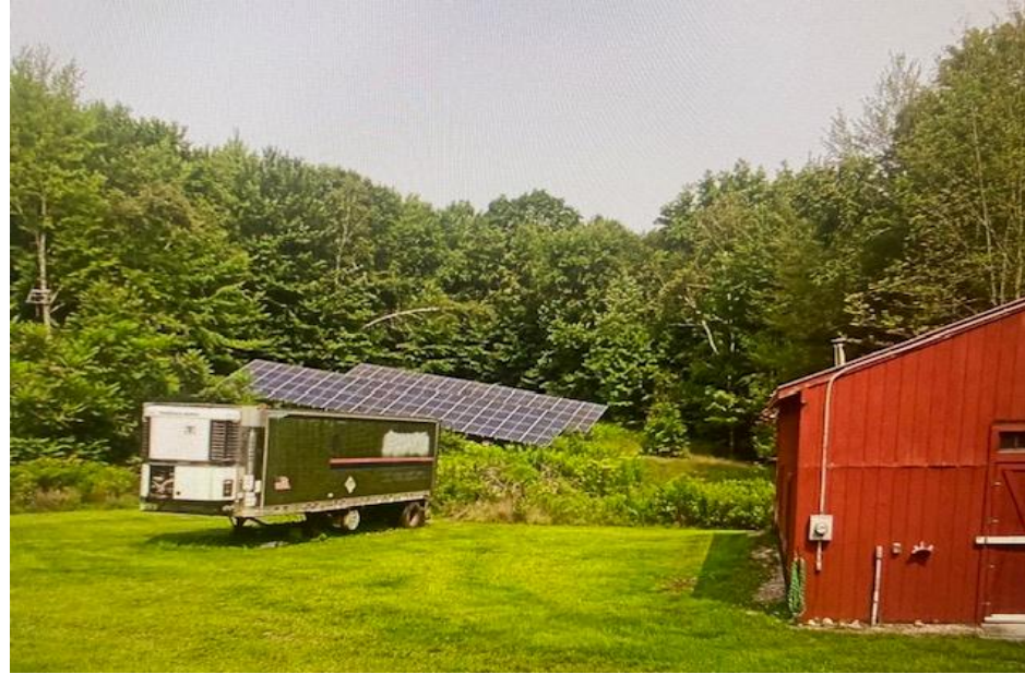
25kW residential solar array
