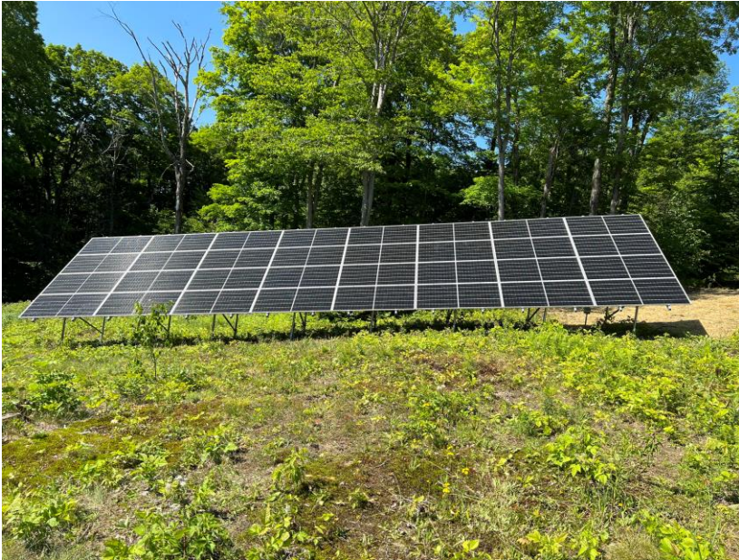
Just under 15kW residential solar array in Barnard
