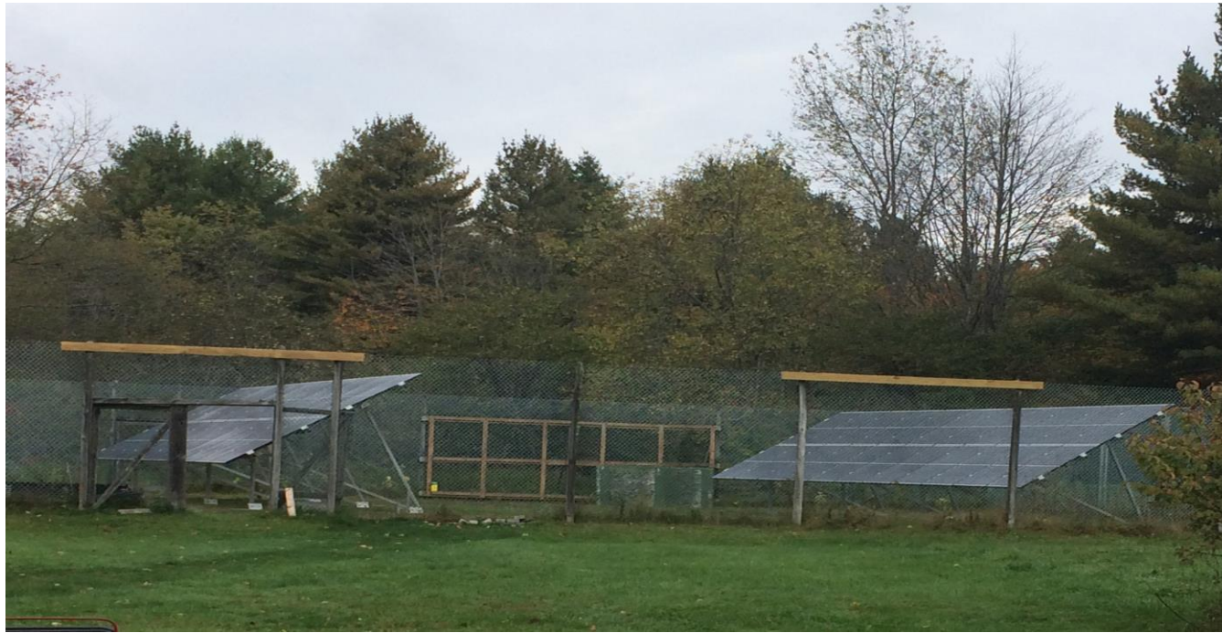
17kW Array in Southern Vermont
