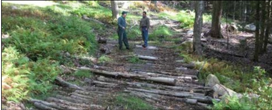
Corduroy on approach to stream crossing. Photo credit: Vermont AMP Manual
