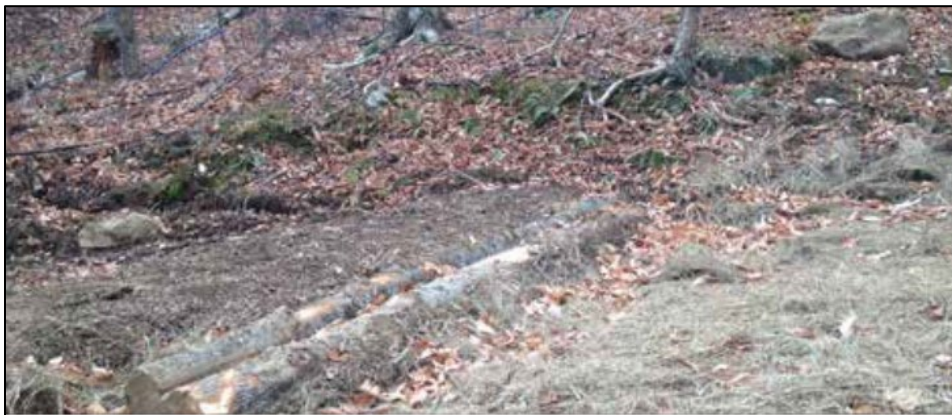
Example of log reinforced water bar on active harvest. Photo credit: Vermont AMP Manual
