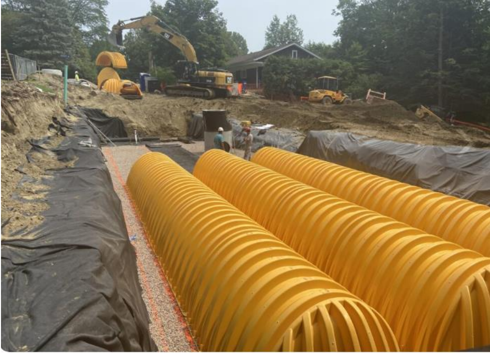
Dry Wells and Detention Chambers
