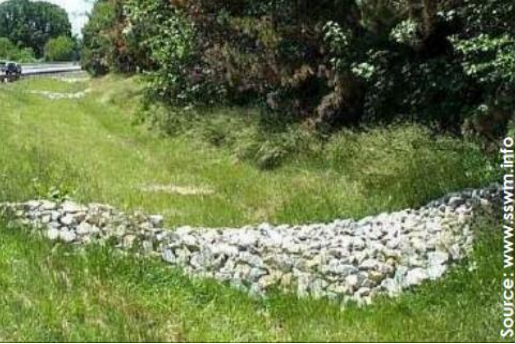
Vegetated Swales, Check Dams
