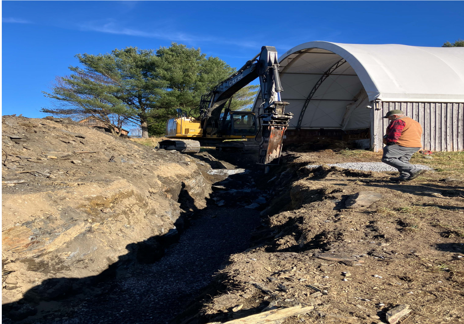
INSTALLATION OF WATER MAIN TO NEW SOURCE TO ADDRESS PFAS CONTAMINATION FOR CRAFTSBURY FD#2 WATER SYSTEM
