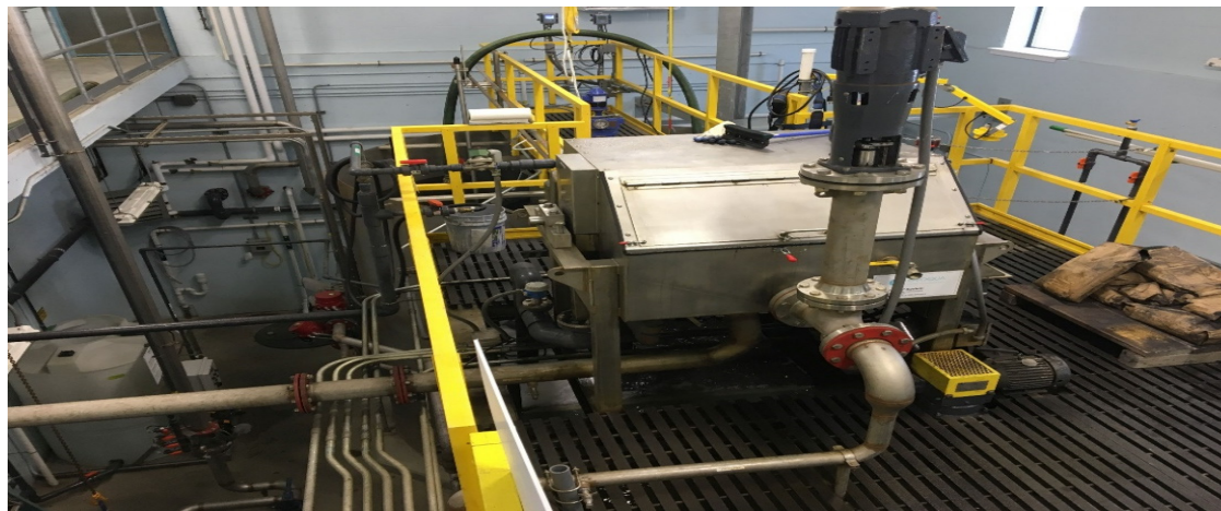
Waterbury WWTF Phosphorus Upgrade: CoMag® process element located within process building.
