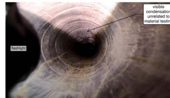
Image 16. Internal wythe, CORE-SOUTH after Goodman Jack testing. Atkinson-Noland & Associates
