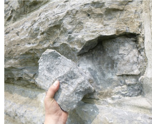
Image 79. Spall removed from the exterior stone masonry. Vertical Access
