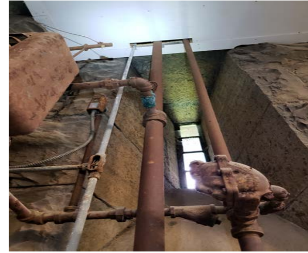
Image 86. Original heating system and piping. Stevens & Associates
