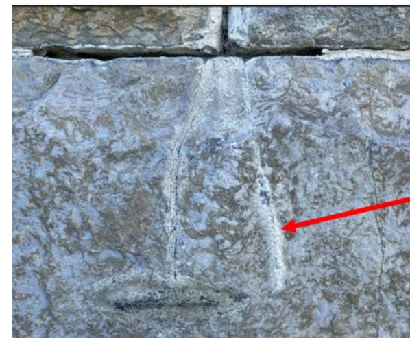
Image 44. White growth along hairline crack. Jablonski
