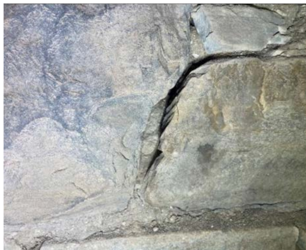
Image 37. Void between two stone units. Jablonski
