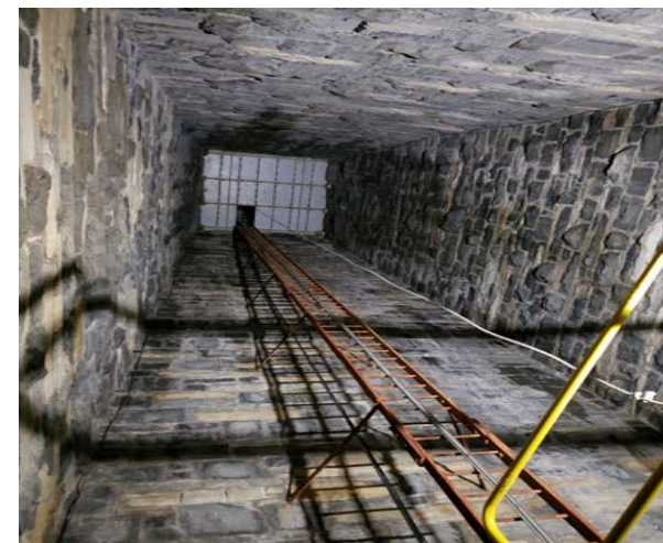
Image 88. Ladder to Level A, above elevator mechanical room. Stevens & Associates
