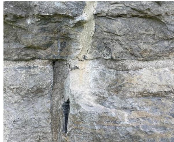
Image 83. Carbonate deposit (White material) below an epoxy crack repair. Jablonski
