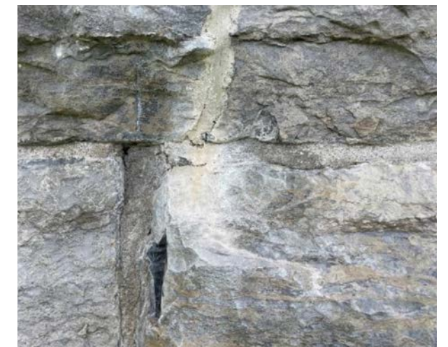
Image 29. Efflorescence and/or carbonate crusts below an earlier caulk repair. Jablonski
