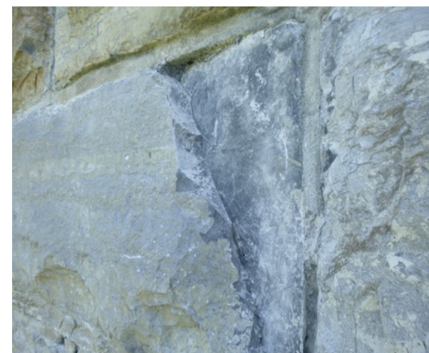
Image 76. Delamination in a stone at the upper portion of the monument. Vertical Access
