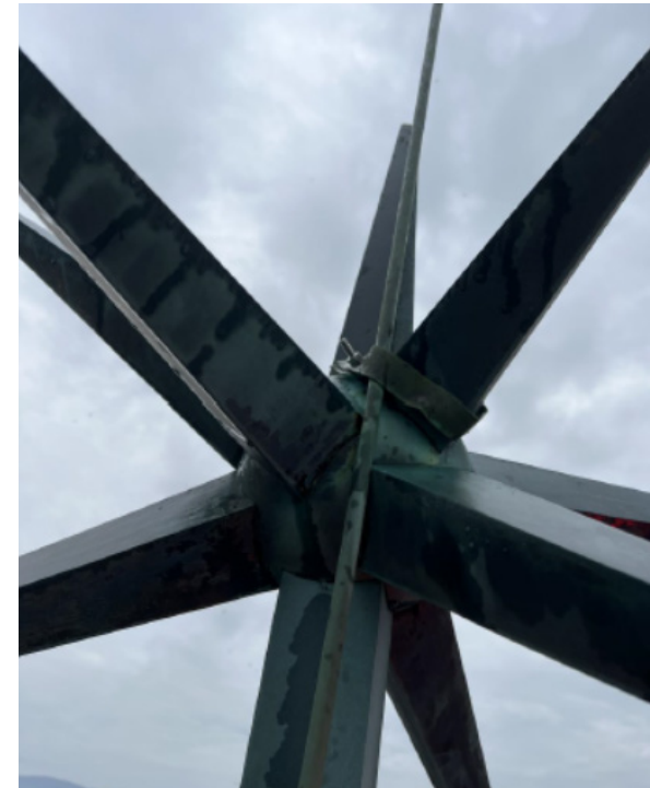
Image 58. 1/2" diameter class II copper air terminal mounted with bolted copper strapping to star finial. Smokestack Lightning.
