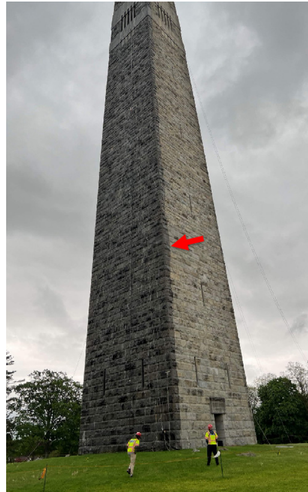
Image 27. North wall following rainstorm with the prevailing wind coming directly from the north. The monument largely blocked wind driven rain from the leeward walls, with a small amount of moisture being blown and wrapping around the corners of the monument creating a clear line of moisture approximately half the length of a stone unit to the East and West elevations.. Atkinson-Noland & Associates
