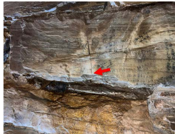
Image 24. Leak observed as a result of spray testing below crack at interior stone. Atkinson-Noland & Associates
