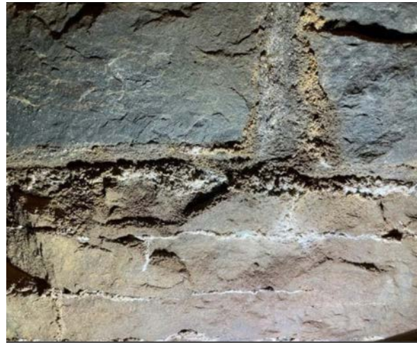
Image 36. Efflorescence and/or carbonate crusts along cracks and mortar joints. Jablonski
