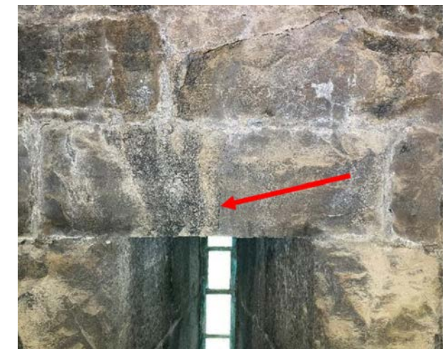
Image 40. Vertical crack running the full height of a window lintel. Jablonski
