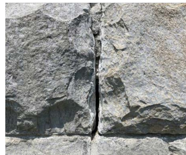
Image 31. Open joint near base of the monument. Jablonski
