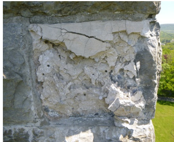
Image 82. Cracked and spalled cementitious patch repair. Vertical Access
