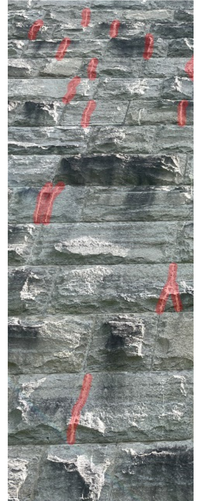
Image 77. Exterior of monument with cracks highlighted in red. Note that most cracks fall below a vertical mortar joint. JBC.
