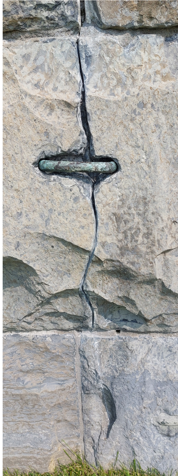
Image 75. Bronze staple condition through crack. Easton Architects
