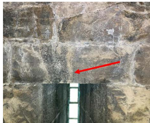
Image 46. Vertical crack running the full height of a window lintel. Jablonski
