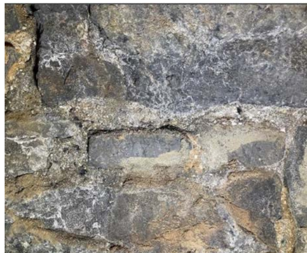
Image 35. Light efflorescence on the surface of the stone units and mortar joints. Jablonski
