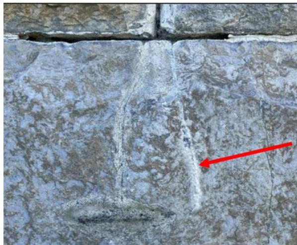
Image 50. White growth along hairline crack. Jablonski
