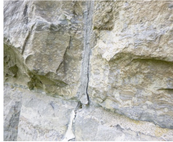
Image 85. Failed mortar joint at upper portion of monument. Vertical Access
