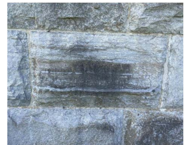
Image 28. Biological growth on surface of exterior stone. Jablonski
