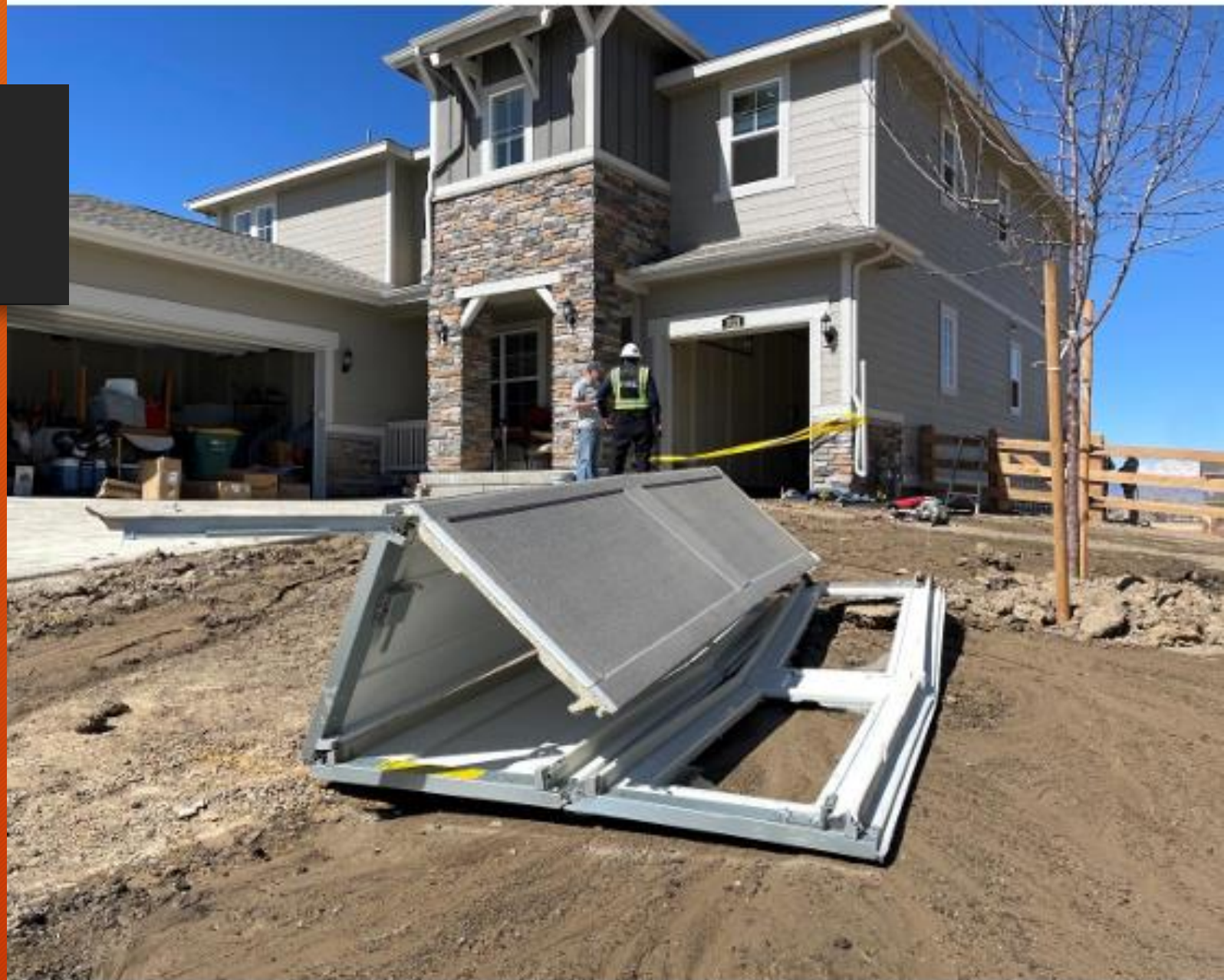
Figure 21 – Garage door location following garage explosion [26].
