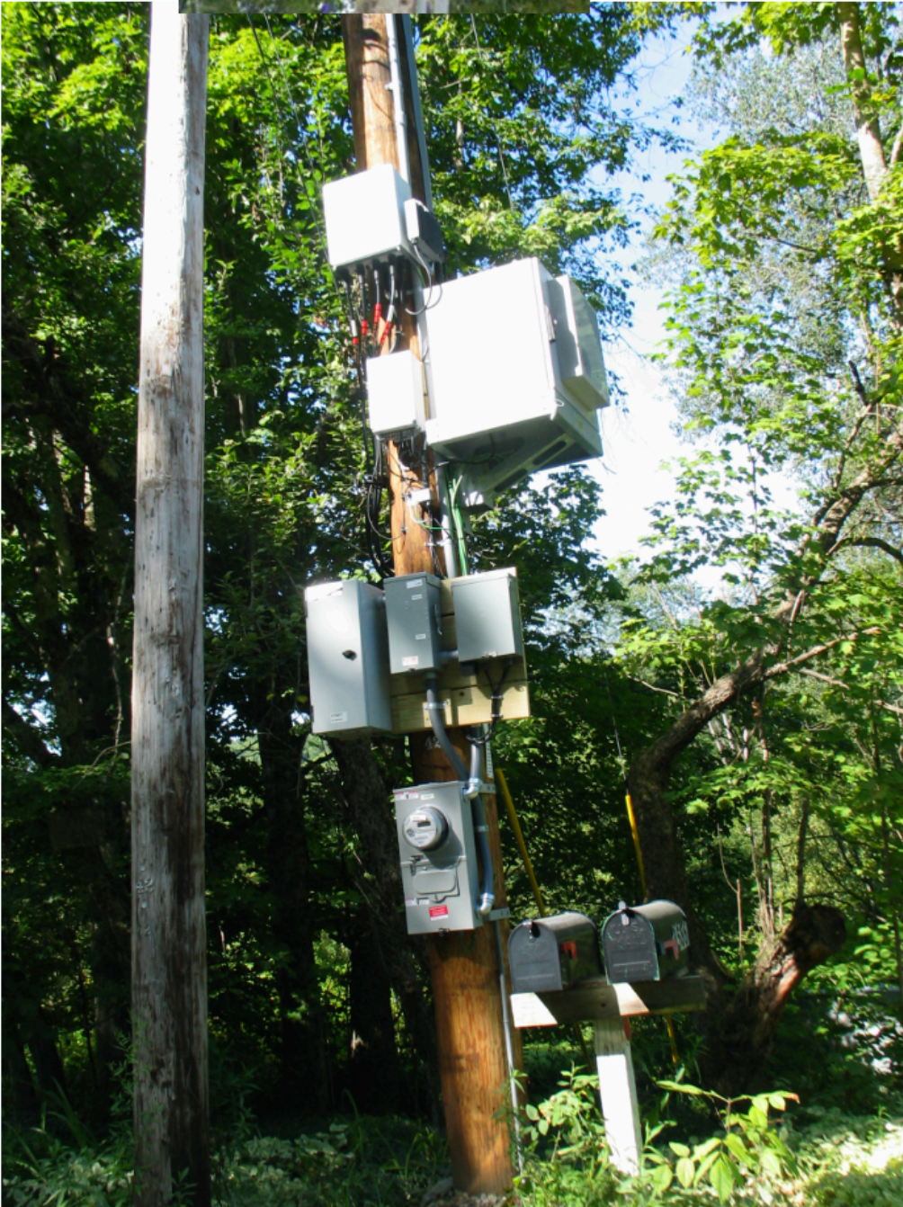
Granville, antenna on pole in residential neighborhood
