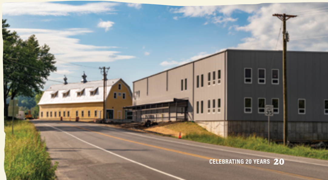
Construction of the Food Hub at the Yellow Barn Complex, June 26, 2024 (Photo: Kelly Bogel Stokes)
