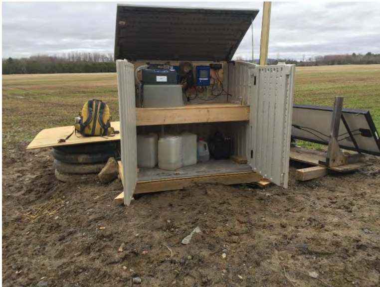
Figure 8. JBT11 monitoring station
