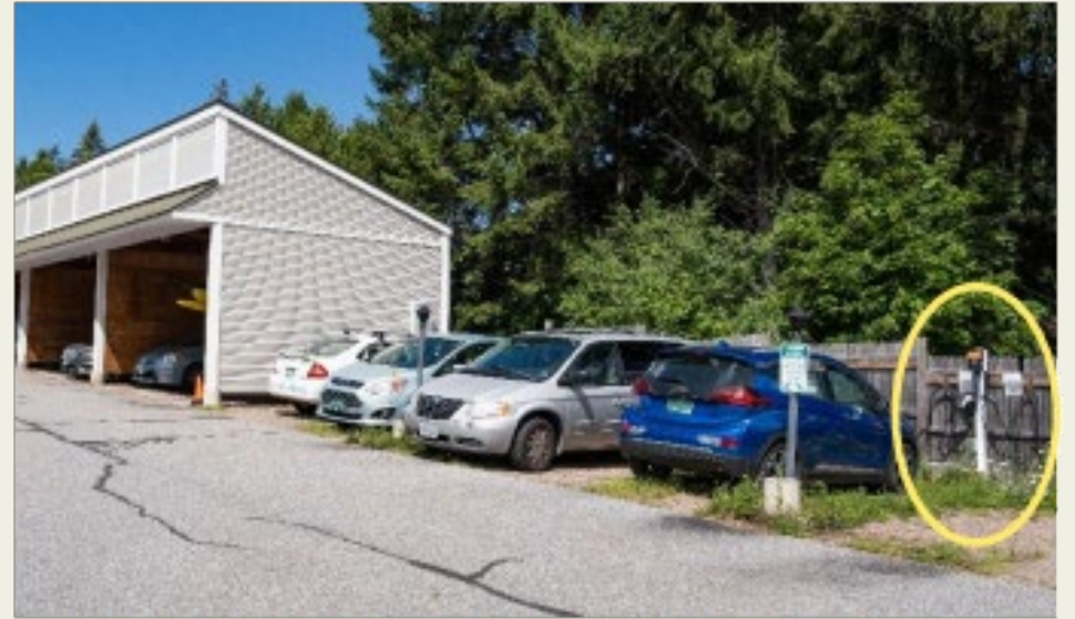
EV charging at Burlington Co-housing East Village Community
