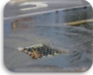
Photo: Road stormwater collection
