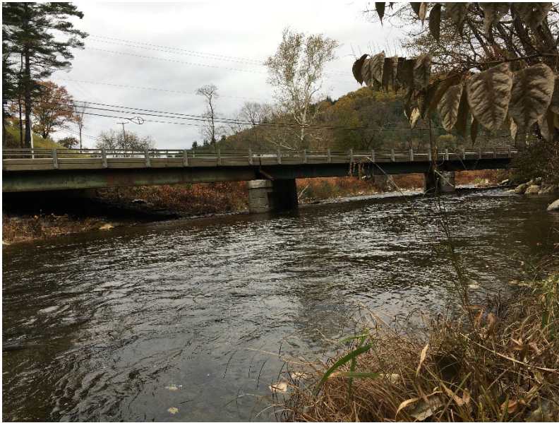
Grafton Bridge 20 on VT 121 Before
