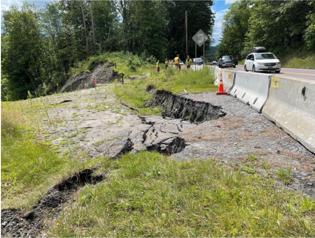
Plainfield, Route 2: Performed subsurface borings, installed instrumentation, developed geotechnical recommendations to stabilize slope and Route 2
