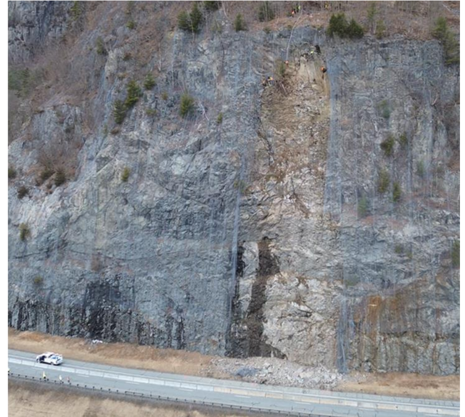
Fairlee, I-91: Large rockfall in February of 2024 that required immediate technical response and emergency repairs
