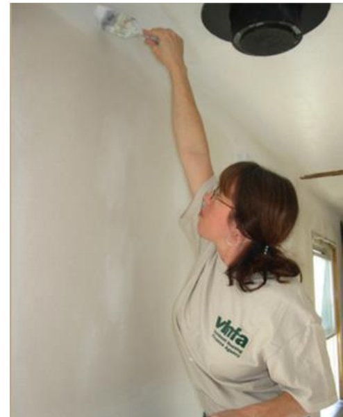
VHFA's Erin Philbrick volunteers with colleagues and Habitat for Humanity at a renovated home in Waterbury.
