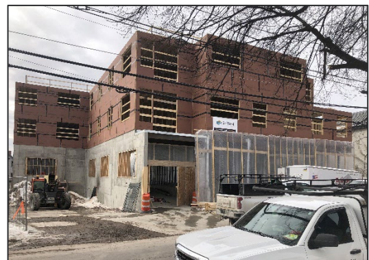
Development of 48 rental units under construction located at 151-157 South Champlain street. Photo provided by the City of Burlington.
