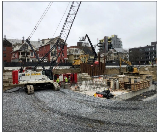
Photos of site preparation of City Place. Photo provided by the City of Burlington
