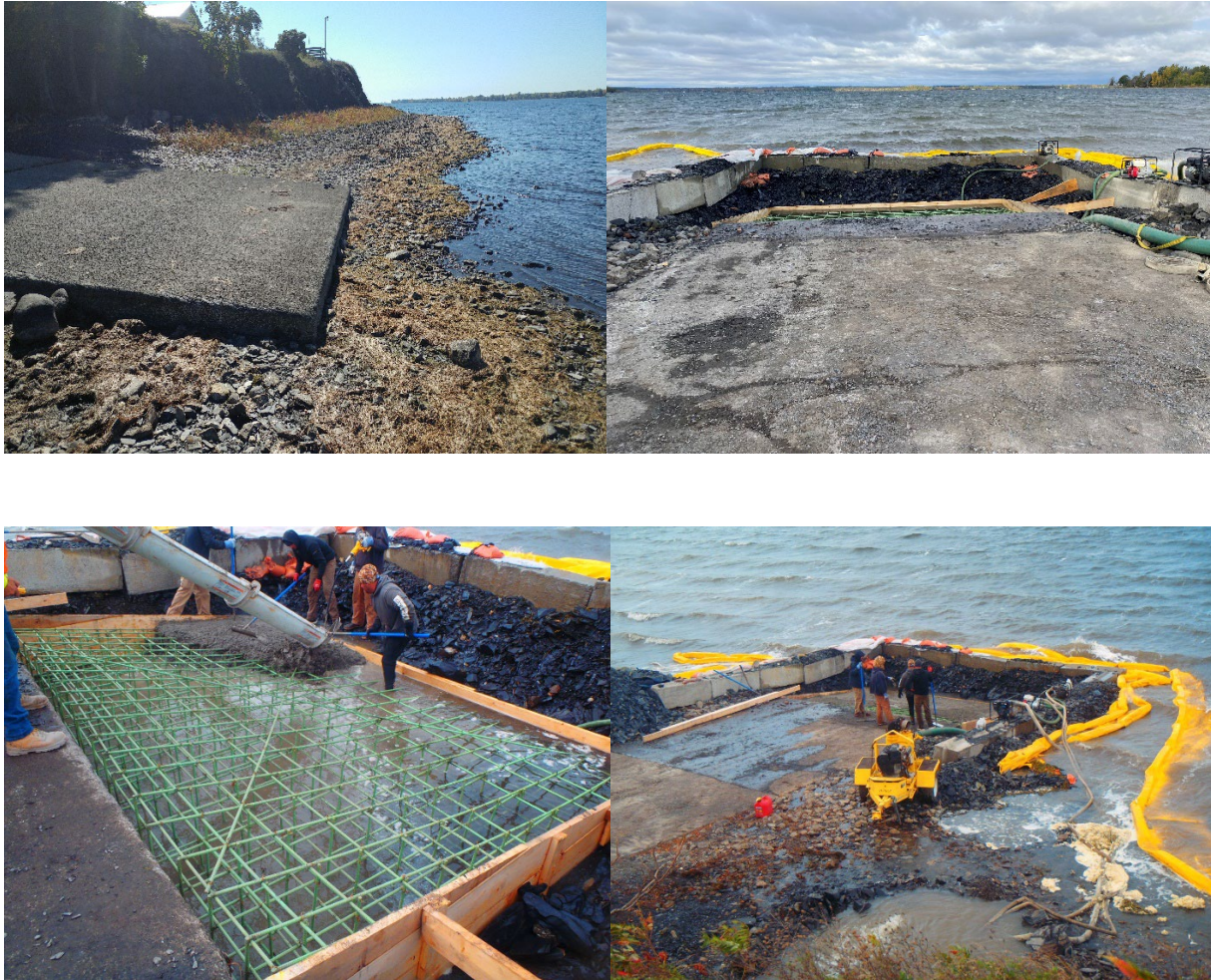
Figure 1. New ramp extension to the Tabor Point Access Area in Swanton on Lake Champlain. From top left (counter clockwise): end of ramp during low water showing a 8 inch drop-off; coffer dam surrounding the end of the ramp; new ramp extension formed and concrete being poured; completed ramp extension with coffer dam and filter curtain.
