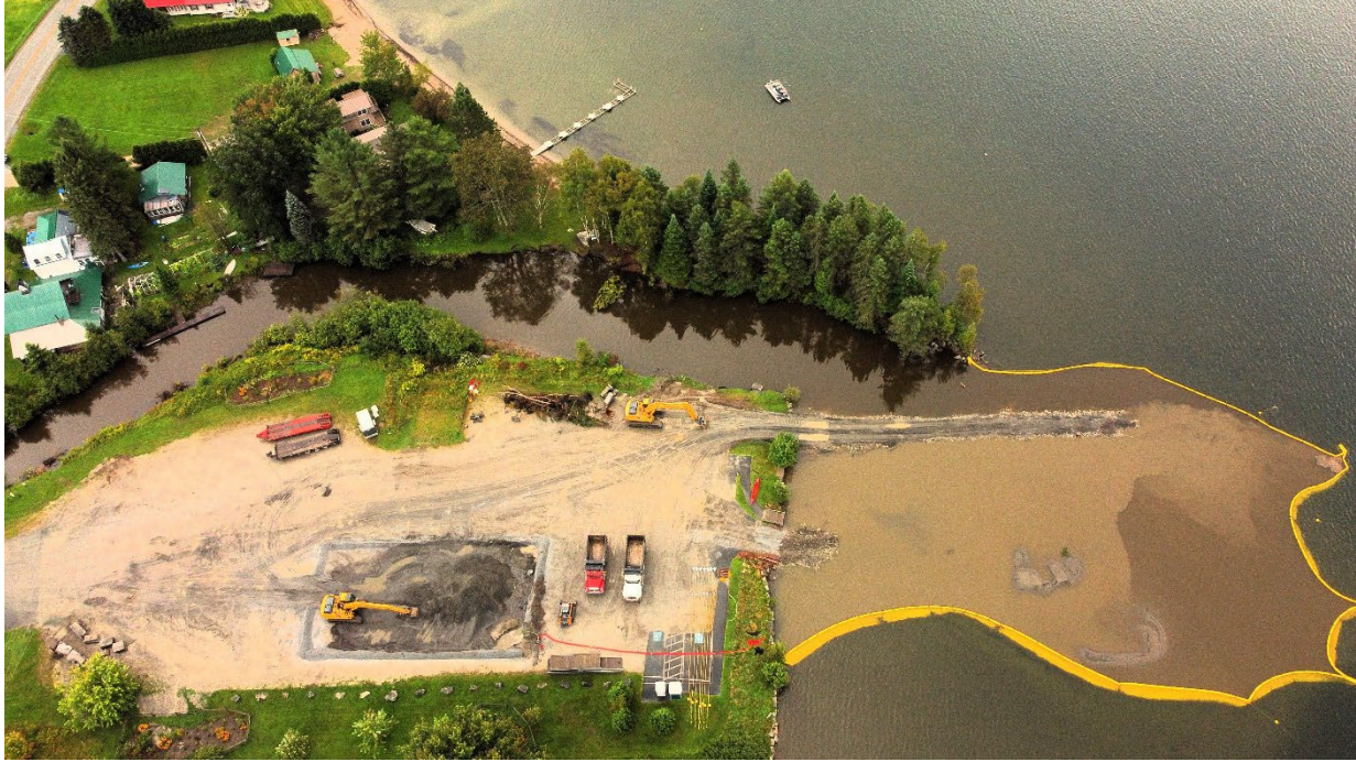
Figure 2. The restoration of the flood damaged Seymour Lake Access Area in Morgan, Vermont. The yellow, in-water turbidity curtain contained all suspended sediment while over 4,500 cubic yards of silt and flood debris were removed from the boat ramp area.
