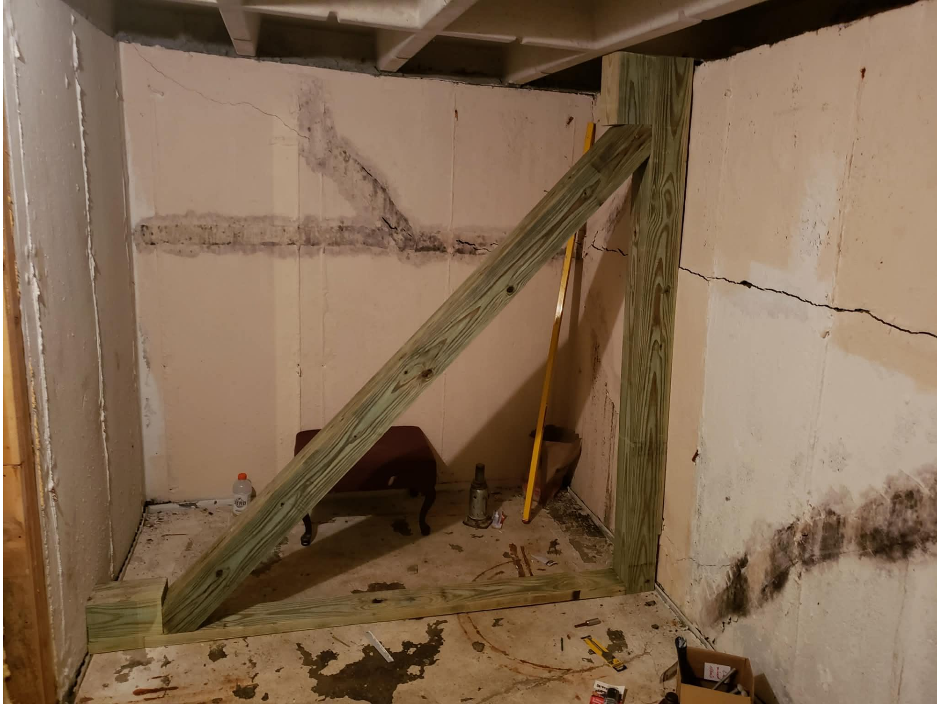
Water and frost heaving damage to south and west basement walls
