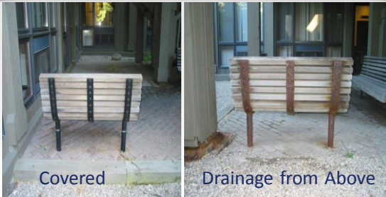
Installed At The Same Time Corrosion Damage
