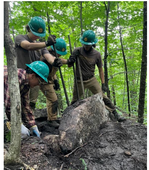
NWSC advanced crews move rocks for a stone staircase on Mtn. Pisgah.
