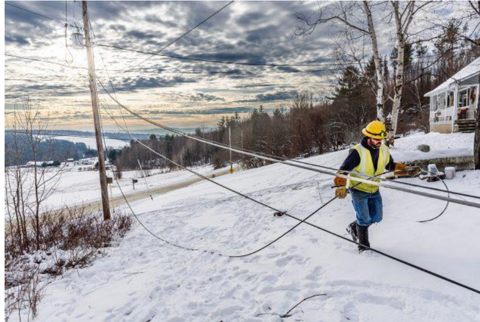
Washington Electric Co-op lineman Donnie Singleton carries part of a downed and de-energized power line, getting ready to splice it. – John Lazenby, The Bridge
