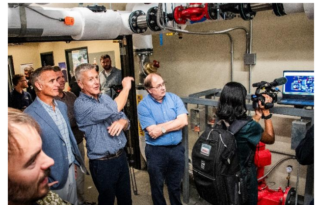
Jay Peak Resort – Dynamic Electrification for main hotel and water park. Reduce 450,000 gallons of propane/year.
