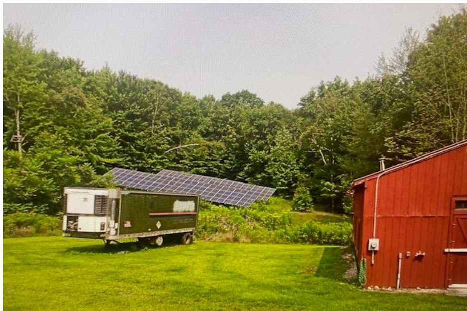
25kW residential solar array
