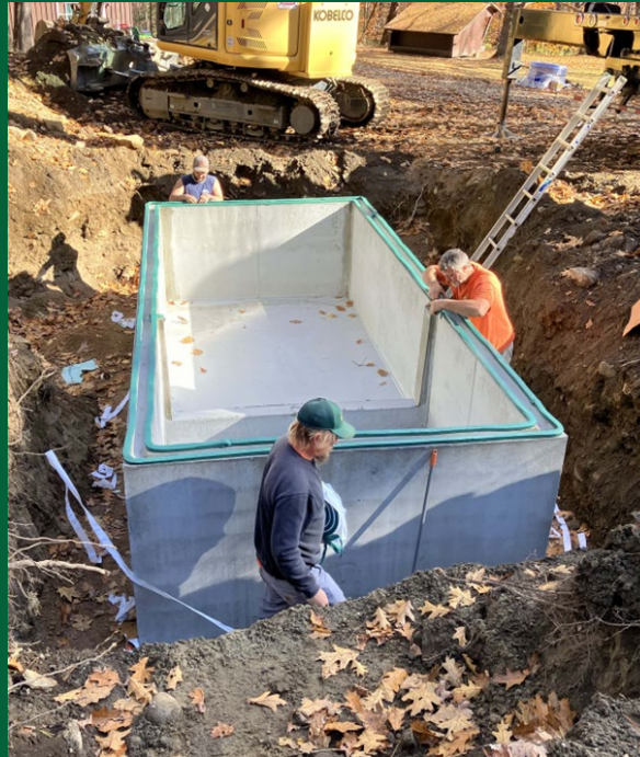
Emergency Wastewater Reserve
