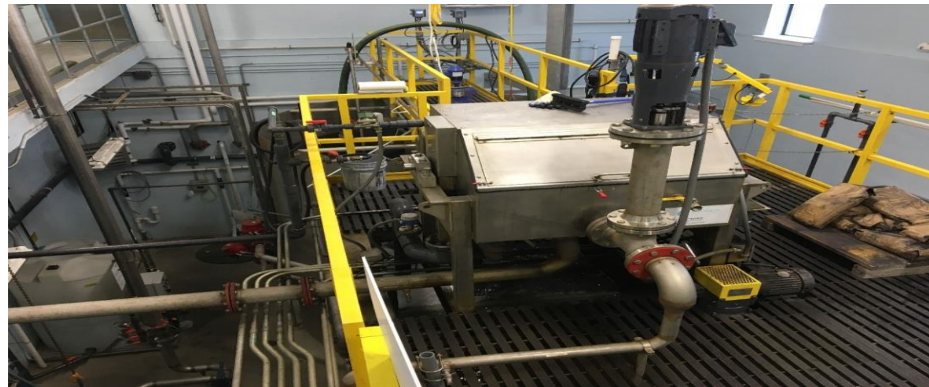
Waterbury WWTF Phosphorus Upgrade: CoMag® process element located within process building.
