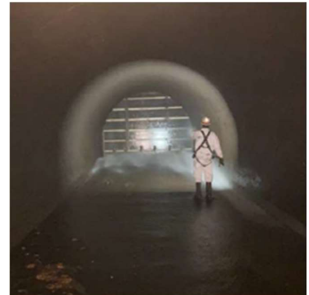
Head Gate in closed position during Fall 2024 pre-cleaning entry
