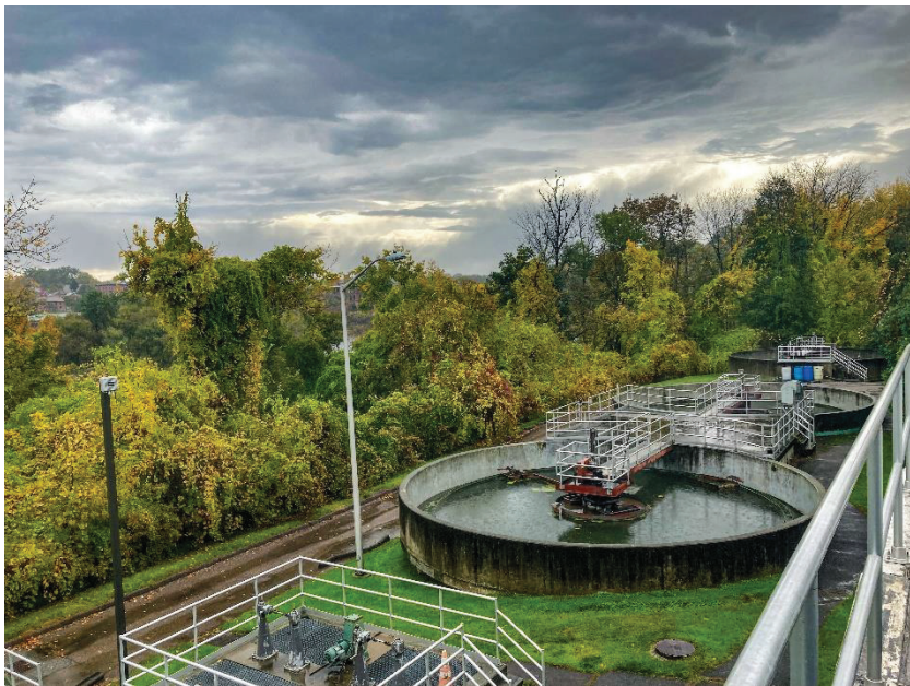
Figure 20: One of three wastewater treatment facilities operated by the City of Burlington. The city has partnered with the State of Vermont to finance several municipal wastewater treatment facility improvements and combined sewer overflow abatement projects. Financing this work has been possible in part by the low-interest loans available through the Clean Water State Revolving Fund.
