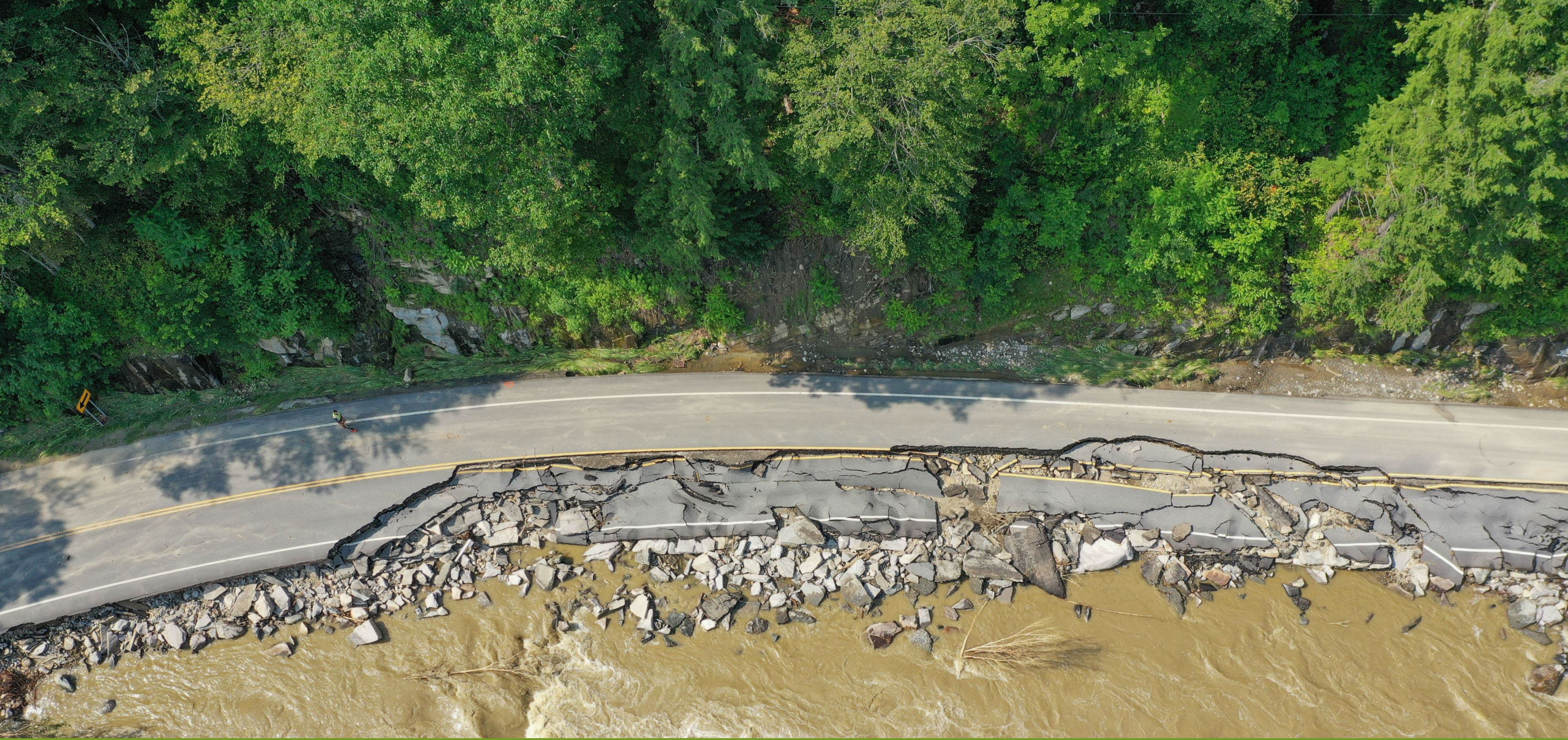
Cavendish VT106 Washout
