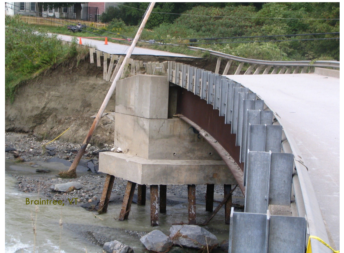
An example of a bridge that was damaged, but the deep foundations allowed the bridge to be repaired and put back in service after TS Irene.
