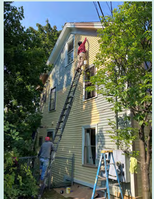
▲ Contractors with VHCB's Healthy & Lead-Safe Homes Program working in Brattleboro. Since 1994, the program has used $35 million in federal funding to improve 2,813 homes.
