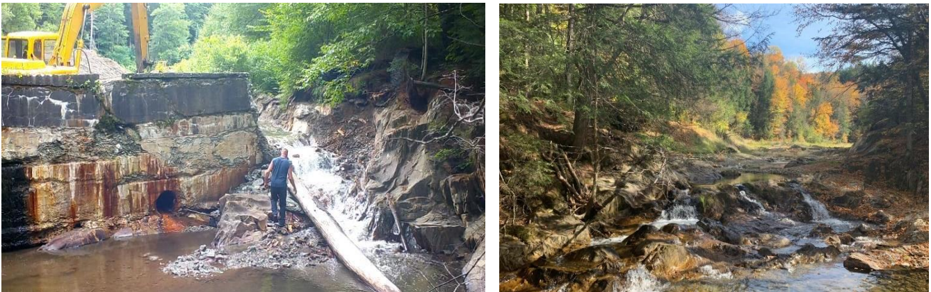
Figure 18. Before (left) and after (right) removal of the Camp Wihakowi dam. Removal of this 100-foot-long concrete dam reconnected 26 stream miles of the Bull Run, a tributary to the Dog River in Northfield, Vermont. The removal was funded by the Department of Environmental Conservation in partnership with Friends of the Winooski River and completed October 2021.
