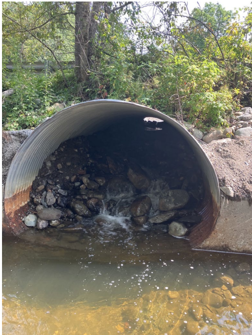
Figure 4: Undersized culverts fail because they have not been sized to pass sediment and debris which are always mobilized by floodwaters
