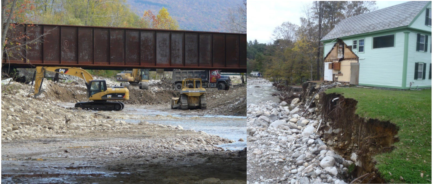
Figure 2: Excessive dredging after floods puts rivers back to an unstable condition ahead of the next flood. More water in the channel equals more stream power equals more destruction to adjacent buildings and infrastructure.
