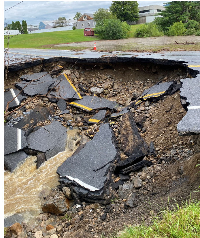
Dow Pond Dam, Middlebury, SIGN Hazard
