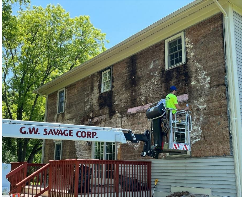
Figure 3. Remediation crew repairing relatively new Vermont home extensively damaged by moisture from indoor air that migrated into the walls (courtesy of Jim Bradley, Hayward Design Build).
