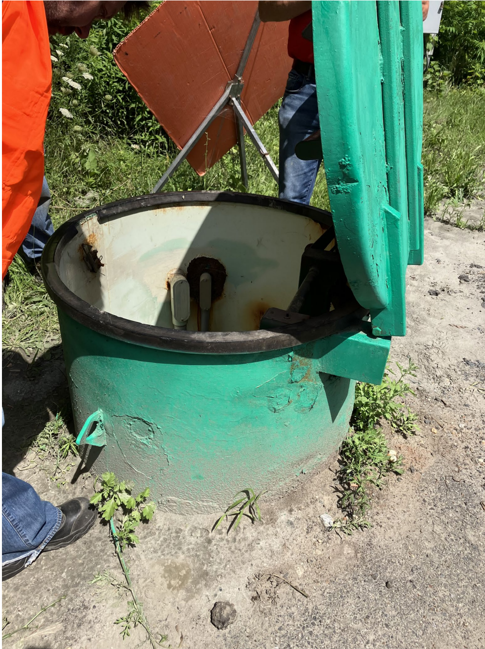
4- Lower State Street Pump Station No.1. Entire Unit was Submerged in Flood Water
