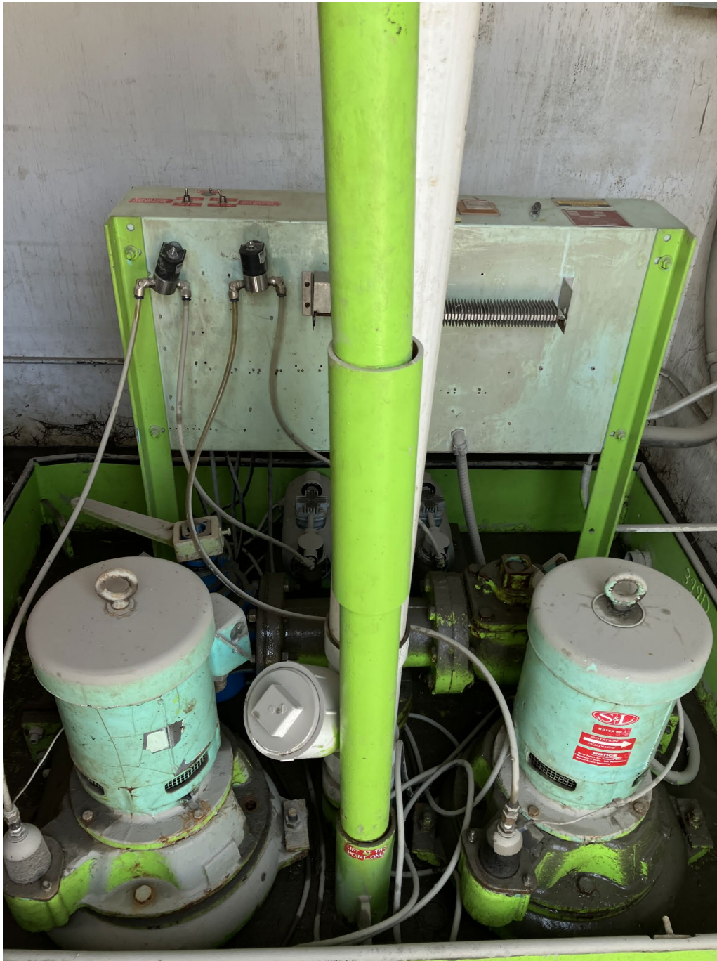
3- Pumps in Lower State Street Pump Station No.2 that Were Completely Submerged in Flood Waters
