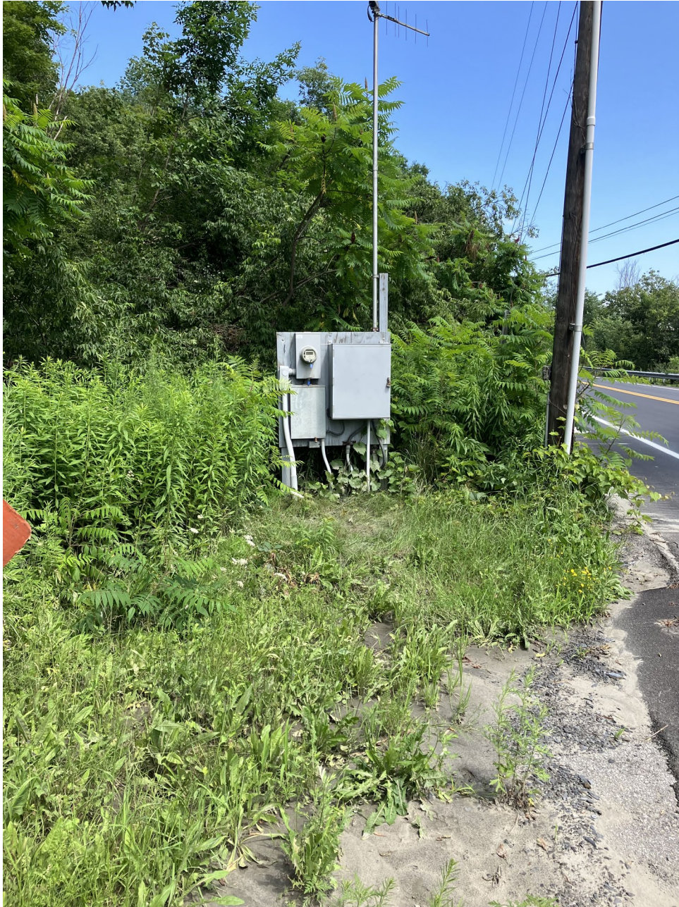
5- Lower State Street Pump Station No.1 Control Panel Which Was Submerged in Flood Water
