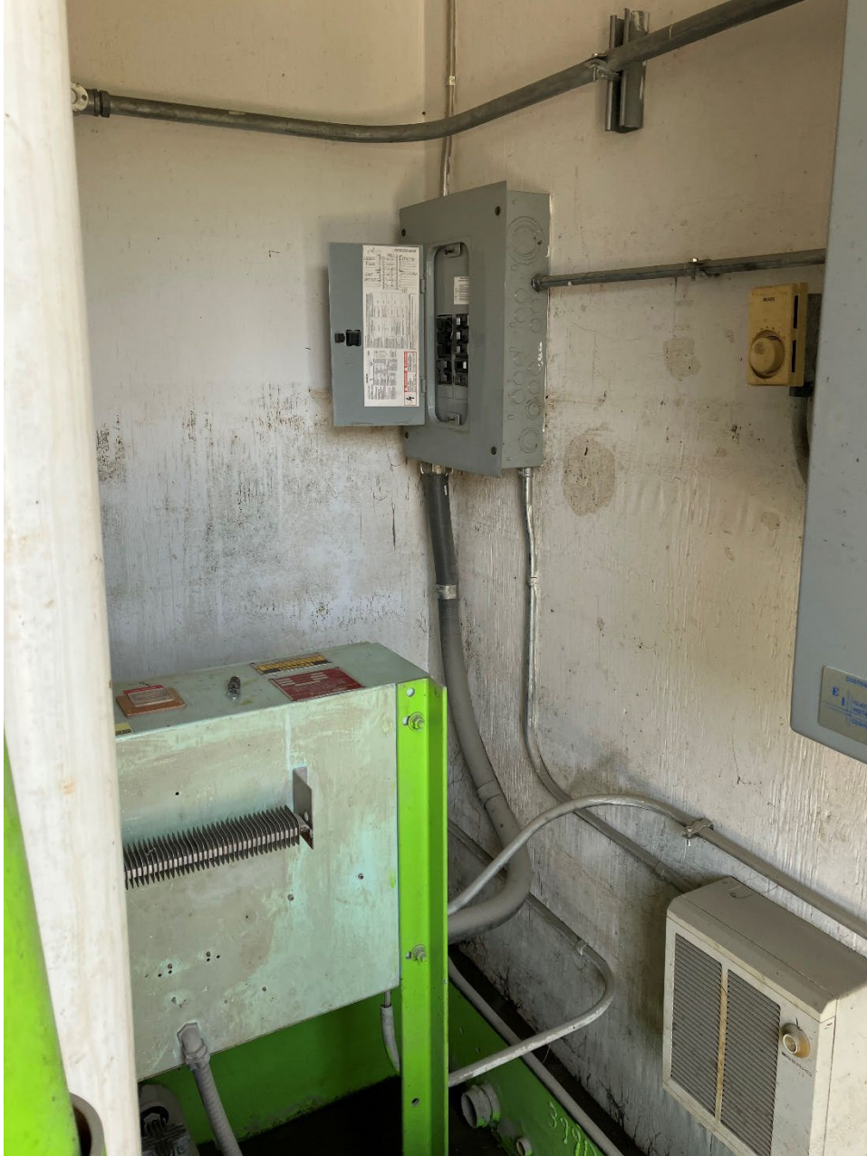
1- Interior of Lower State Street Pump Station No.2. Note Highwater Mark at Approximately 4 Feet
