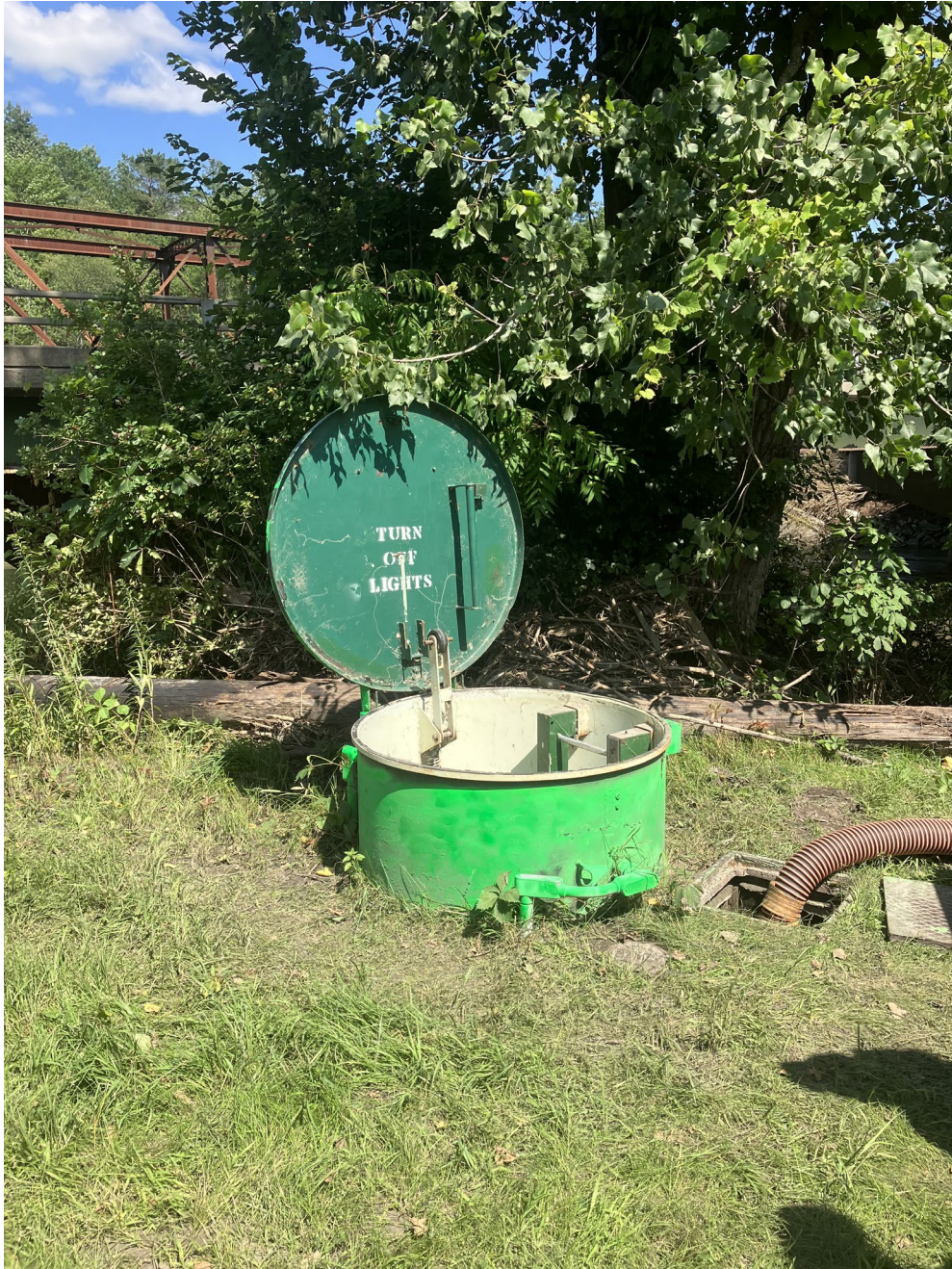
6- Interstate Equipment Pump Station No.4 Entire Unit Was Submerged in Flood Water
