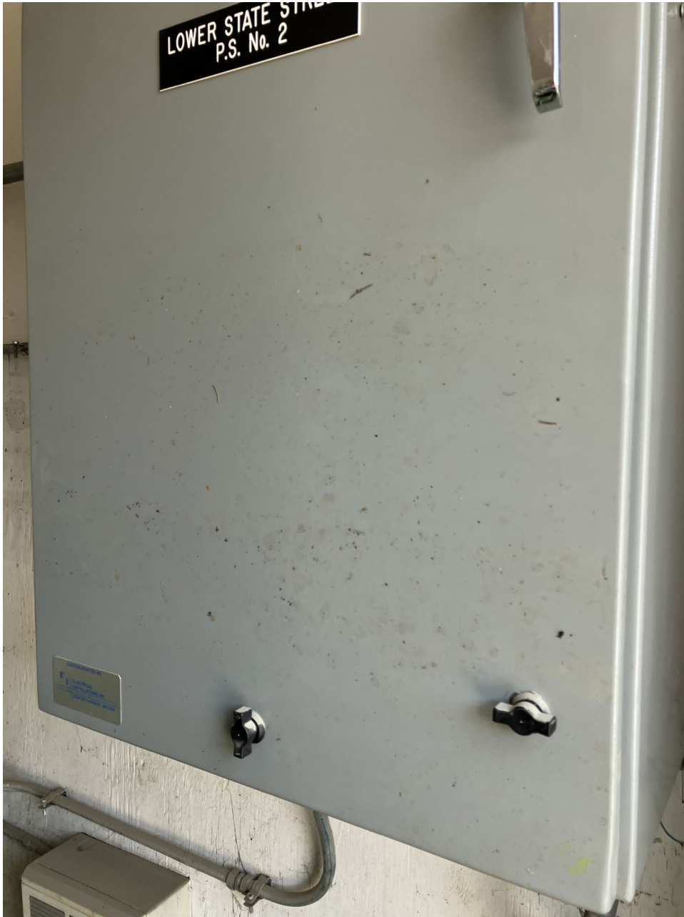
2- Control Panel of Lower State Street Pump Station No.2. Note Highwater Mark at Approximately 4 Feet
