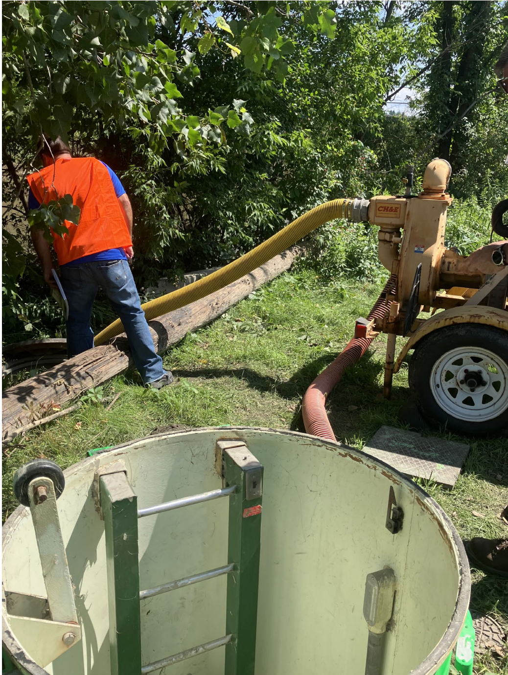
7- Interstate Equipment Pump Station No.4 With Portable Pump Being Used
