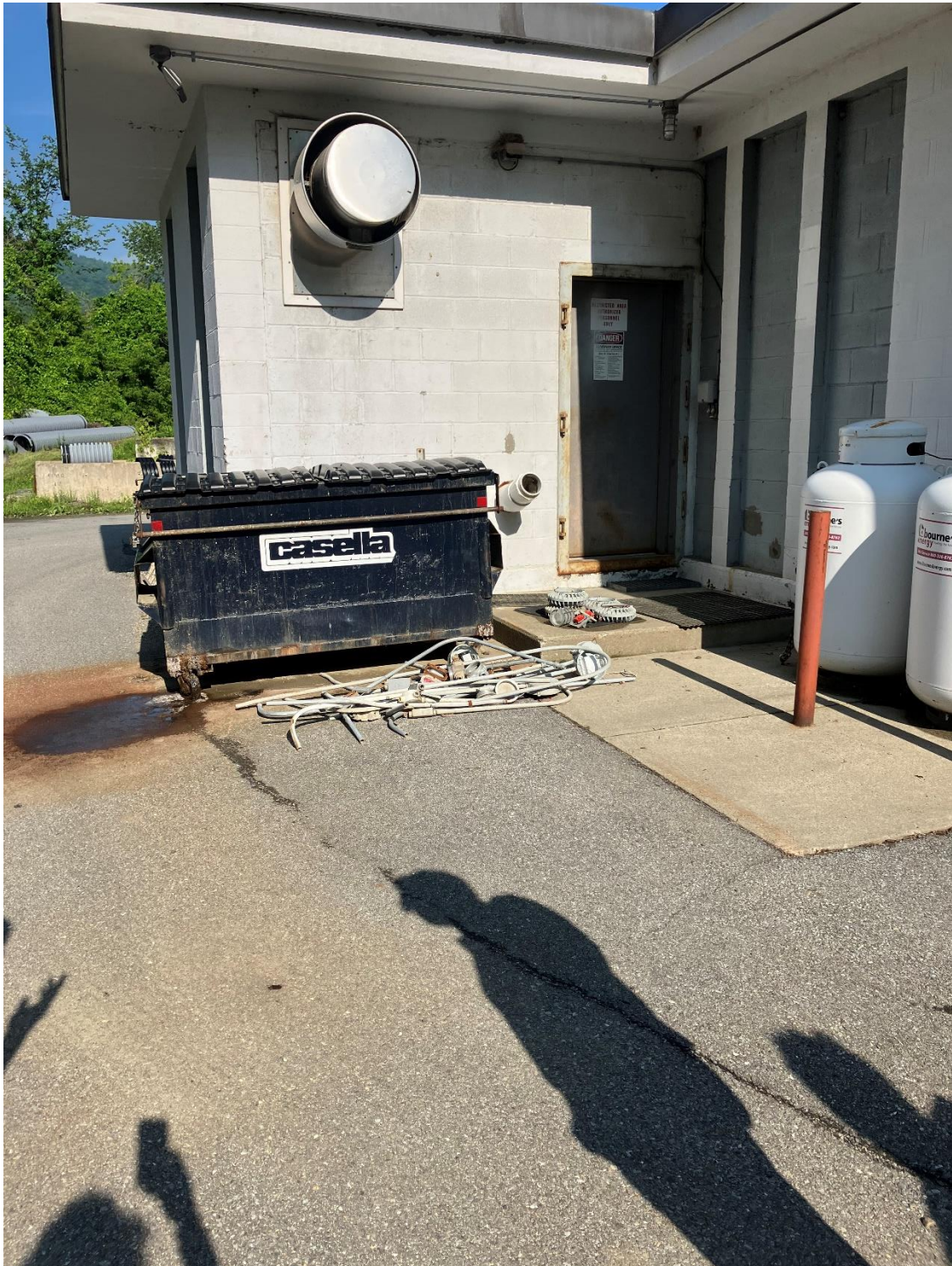
11- Main Street Pump Station Exterior. Showing Damaged Electrical Components in the Process of Being Removed.
