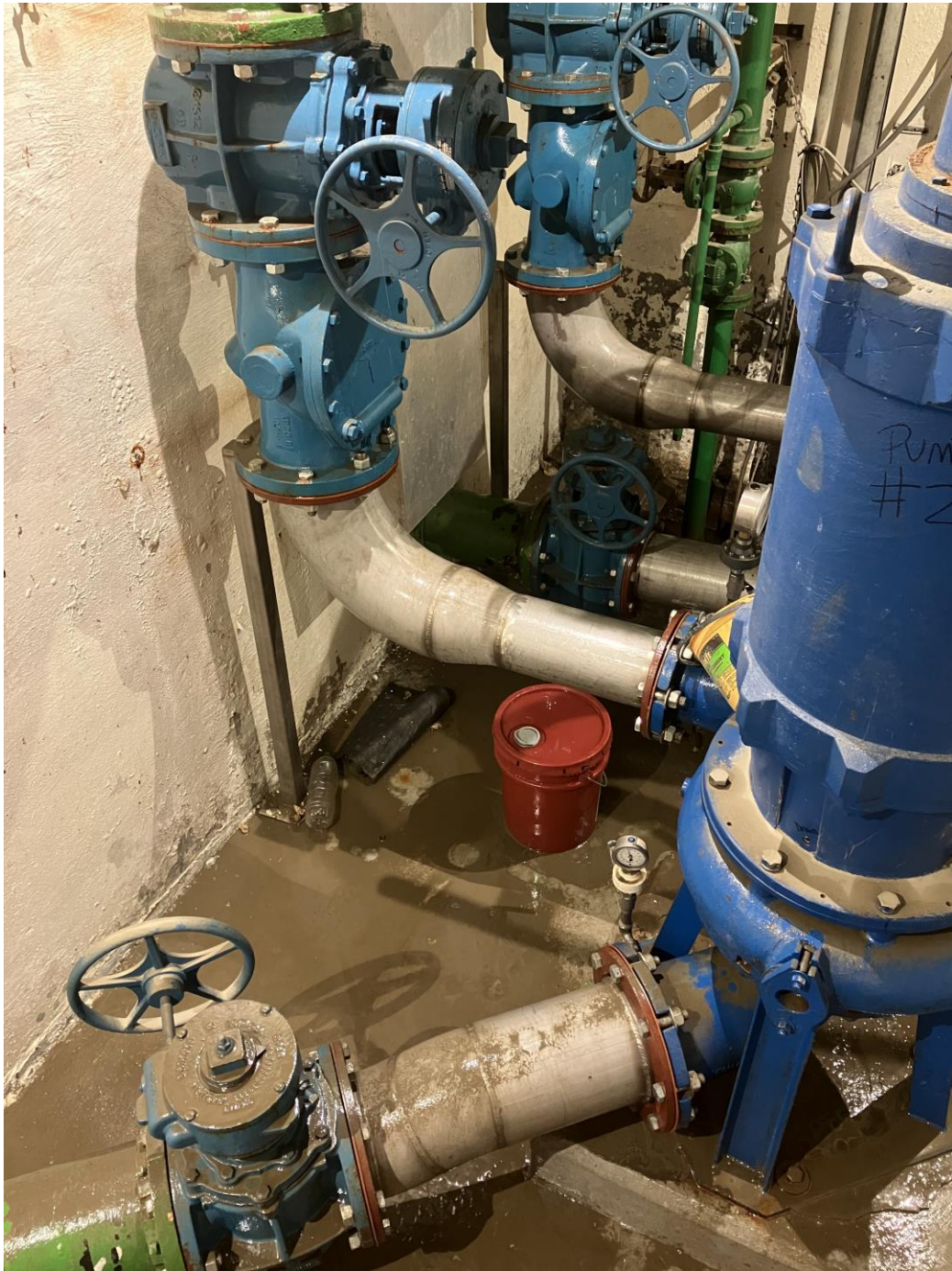
9- Main Street Pump Station Basement Level. High Water Mark Was Approximately Feet, But Water Had Leaked Down from Upper Levels and Was in Contact With Upper Portions of the Pumps
