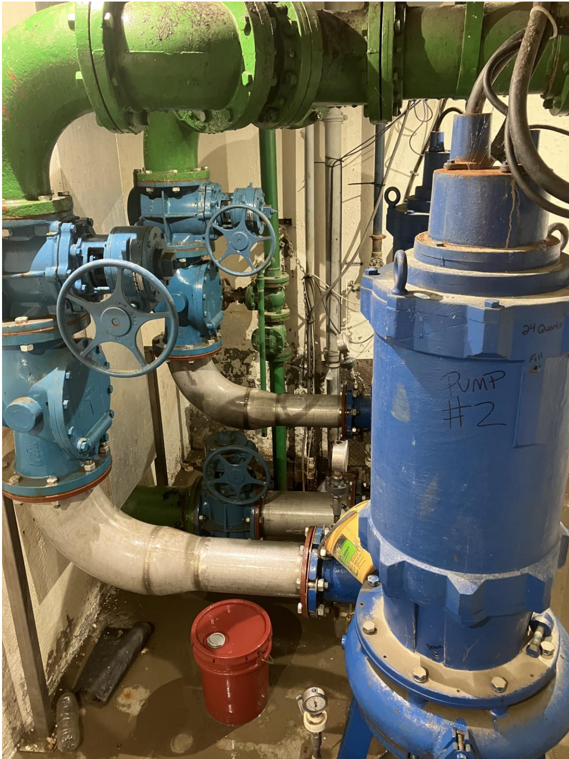
10- Main Street Pump Station Basement Level. Showing Silt on Top of Piping from Leaking Down from Upper Levels
