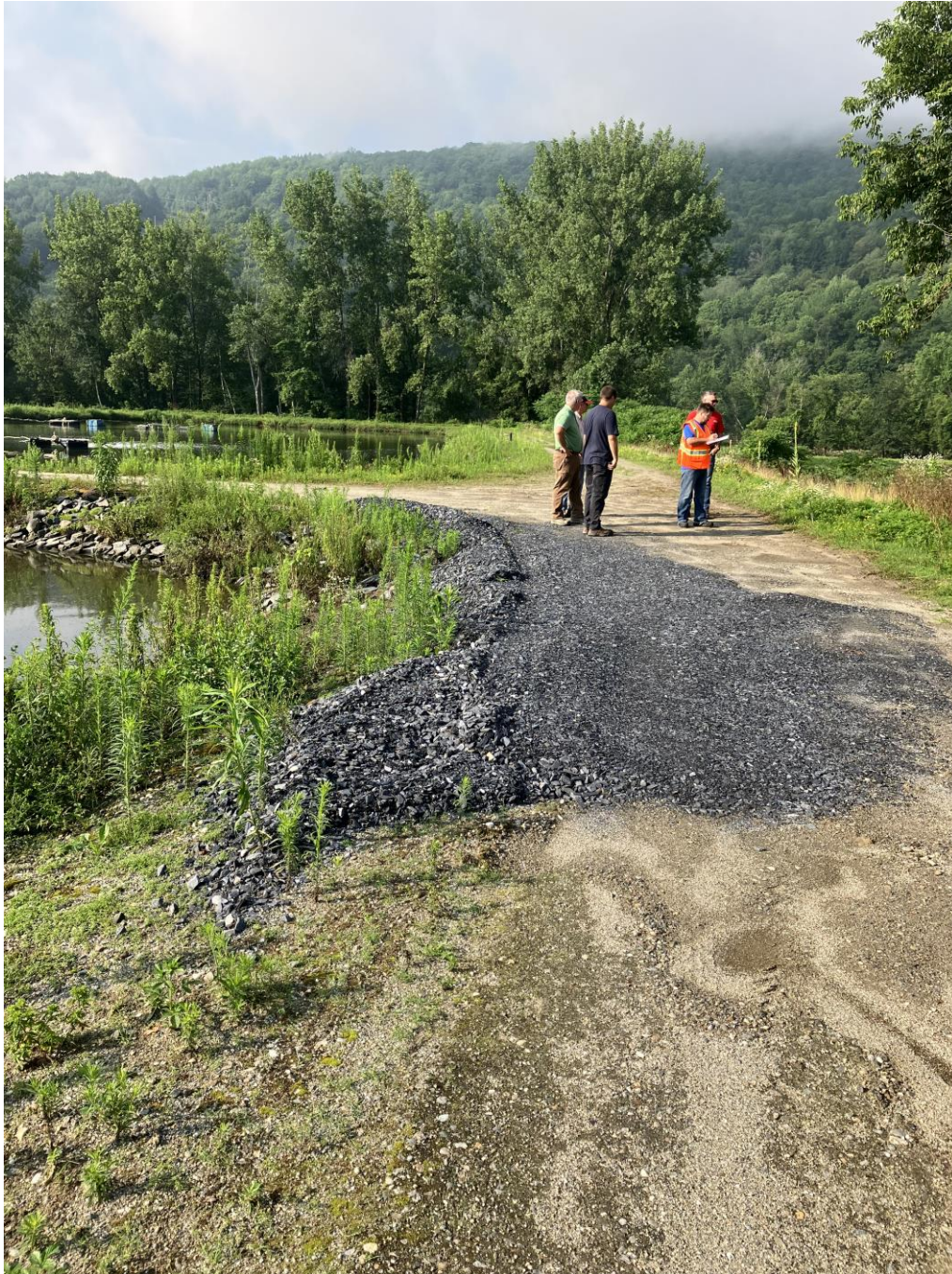
7- View of Backside of Lagoon 1 After Flood Waters Had Receded July 19,2023. Fill Material Was Added During the Flood Event to Prevent the Lagoon from Overflowing
