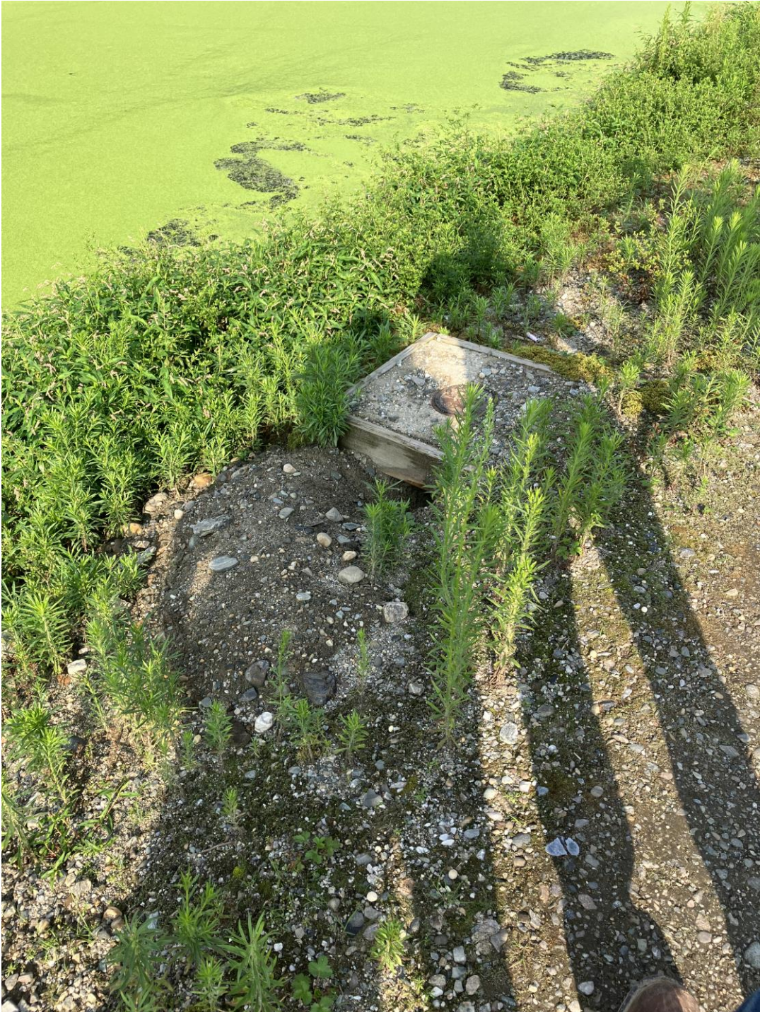
5- Erosion Near Berm of Lagoon 3
