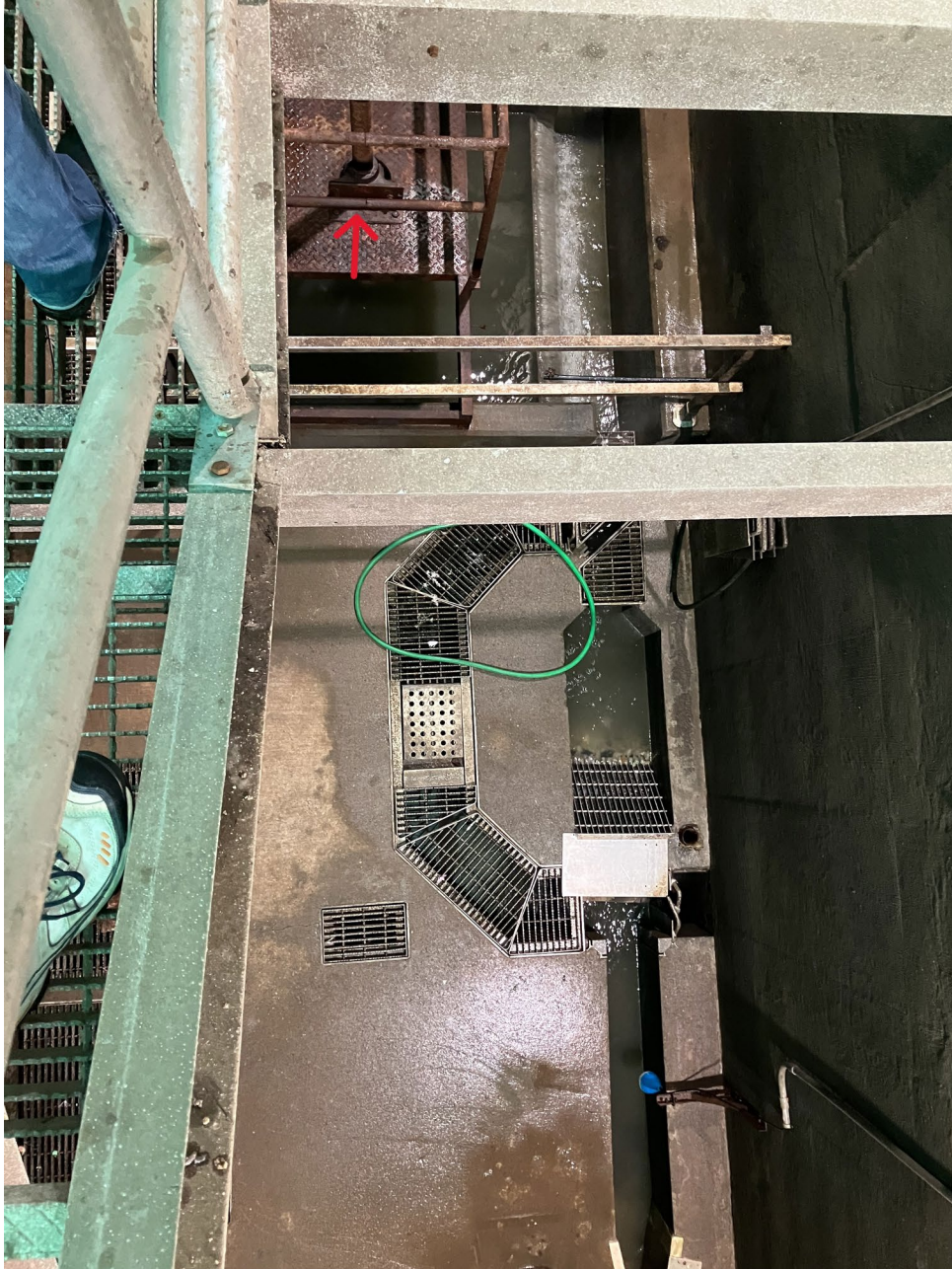
4- Grit pump in Main Pump Station
