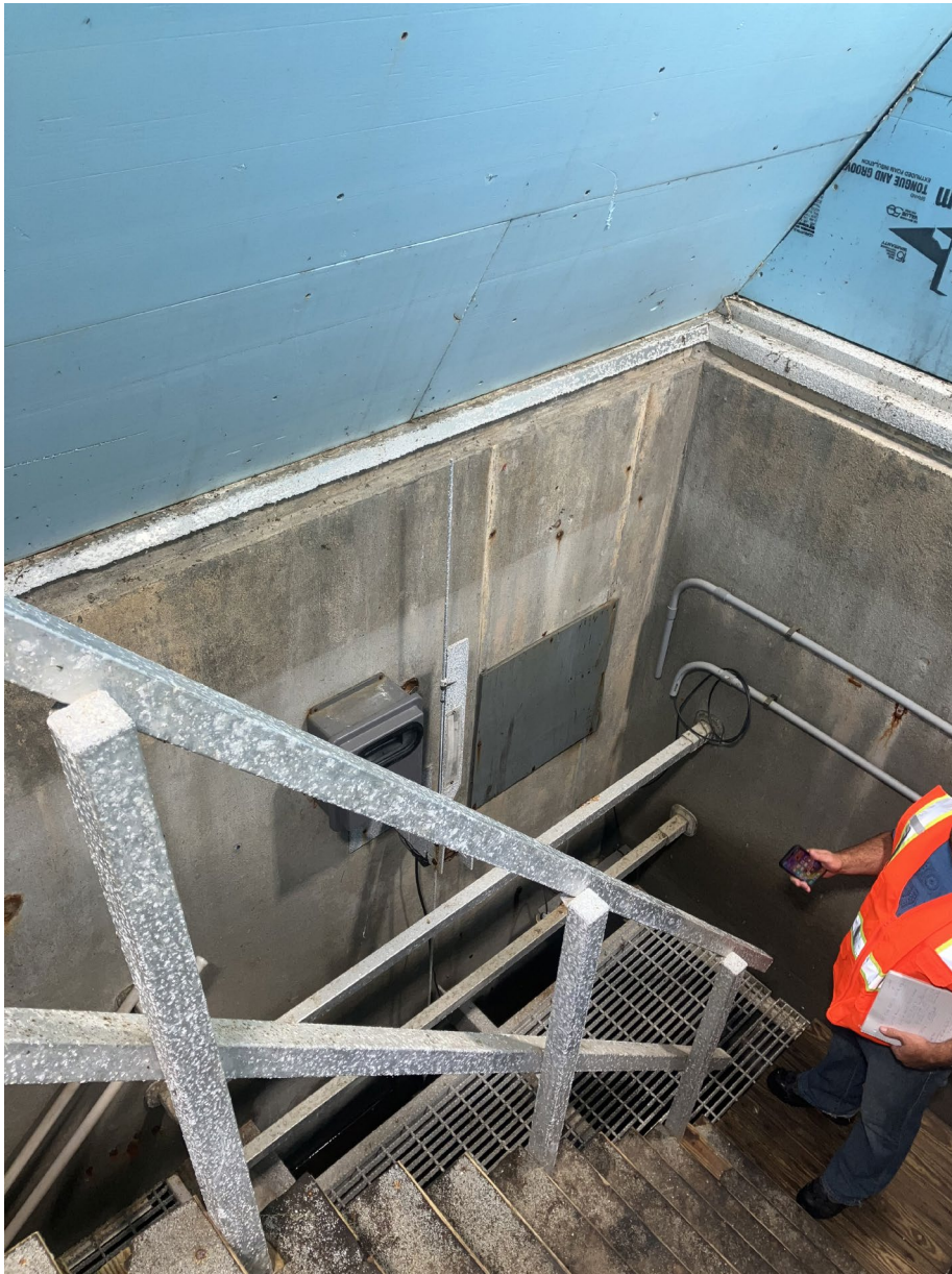
1- Old Flow Meter (Note Flood Water Line Was 12 Inches Above Meter as Depicted by the Lighter Gray Line on Wall)
