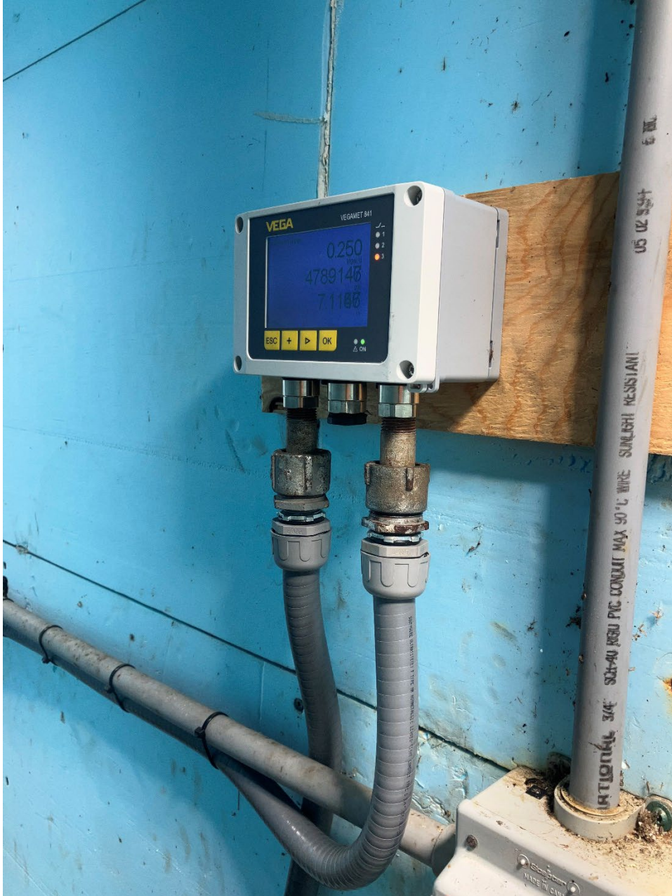
2- New Flow Meter Elevated to Above Grade Just Inside the Doorway of the Outfall Building
