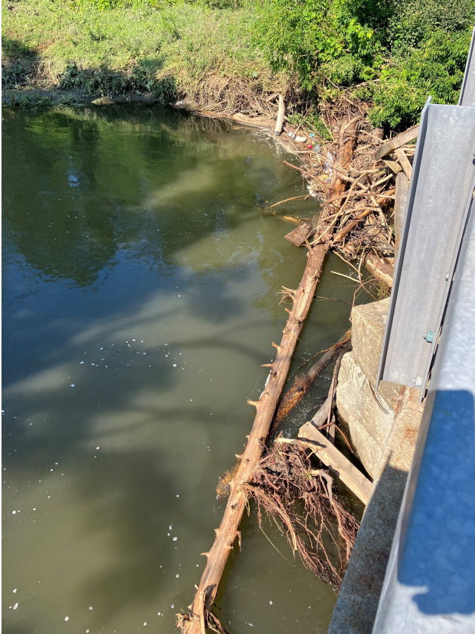
5- Bridge Above Submerged Sewer Line Under the River. Manholes are Located on Both Sides of the River
