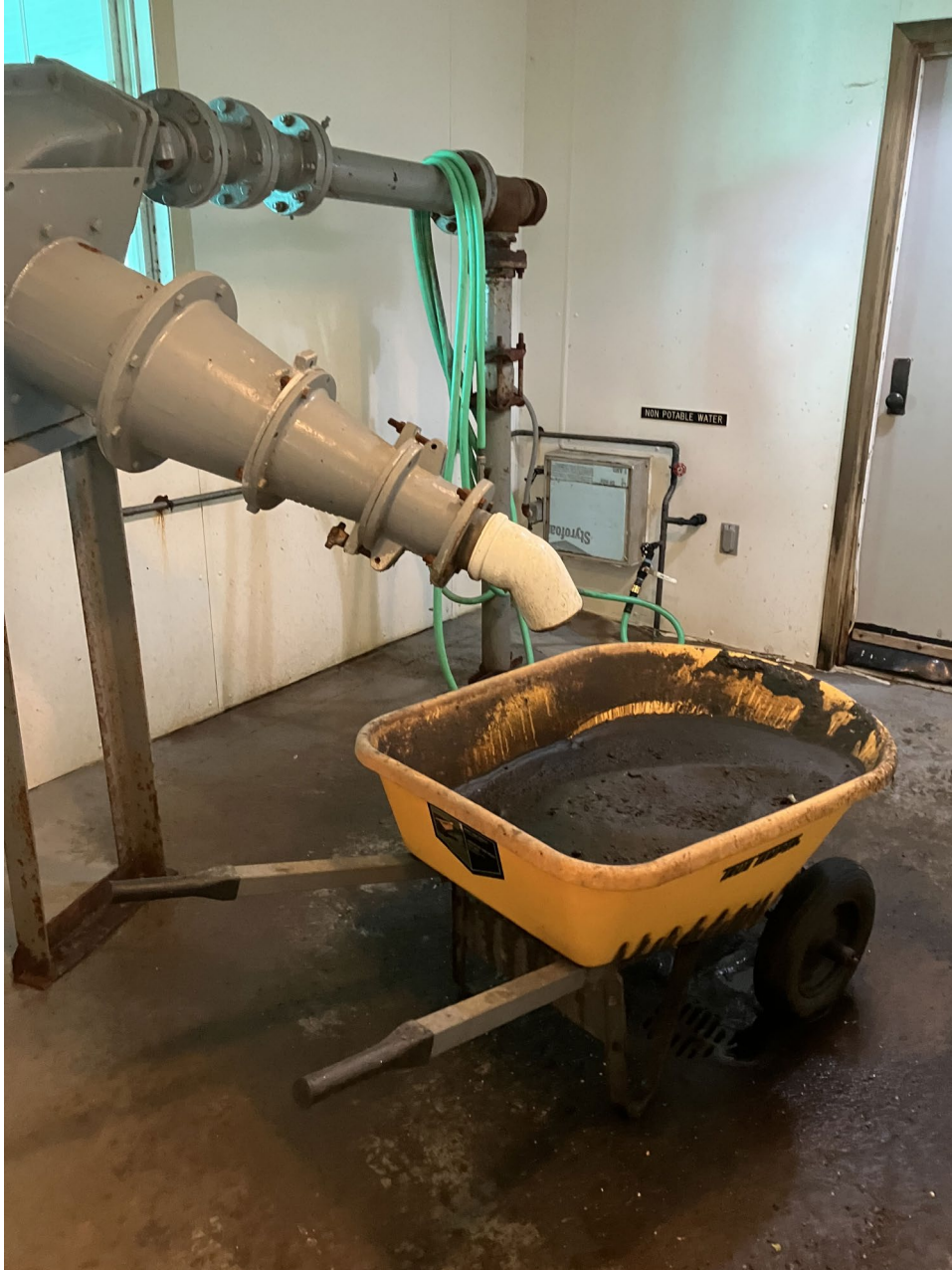
5- Excessive Grit from Grit Pump in Main Pump Station
