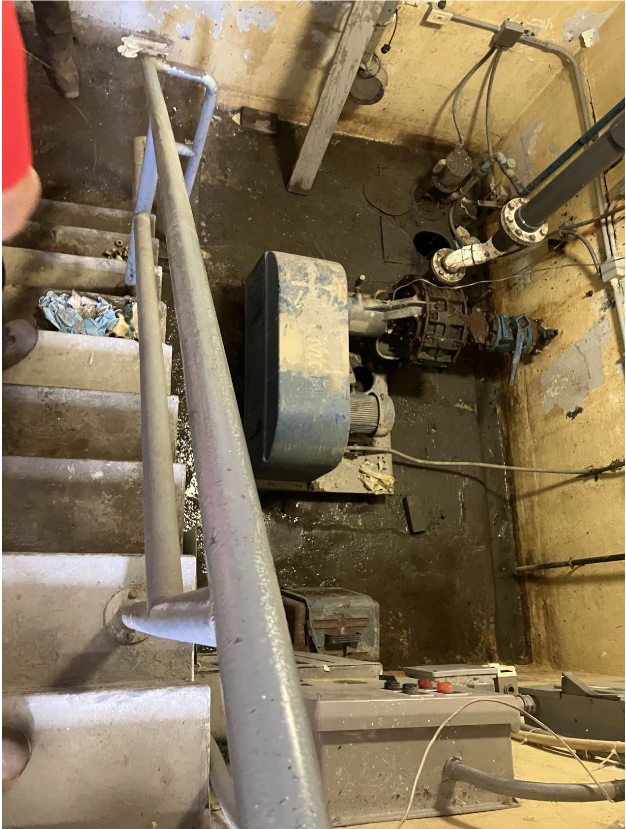
Grit pump room
