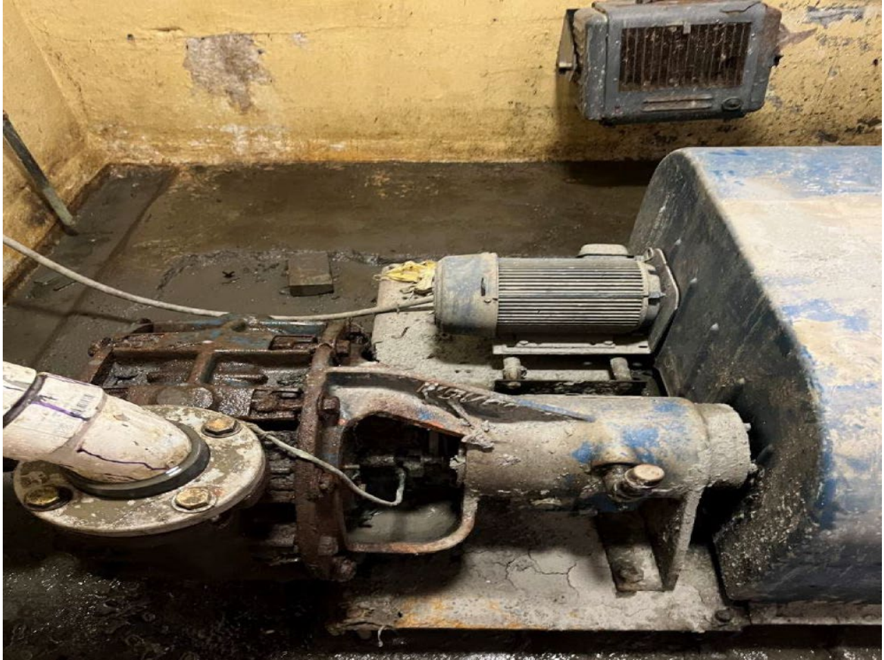
Grit pump & heater
