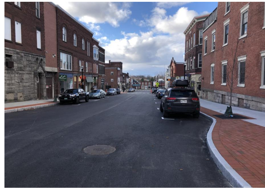
Reconstruction of Kingman Street. Photo Provided by the City of St. Albans
