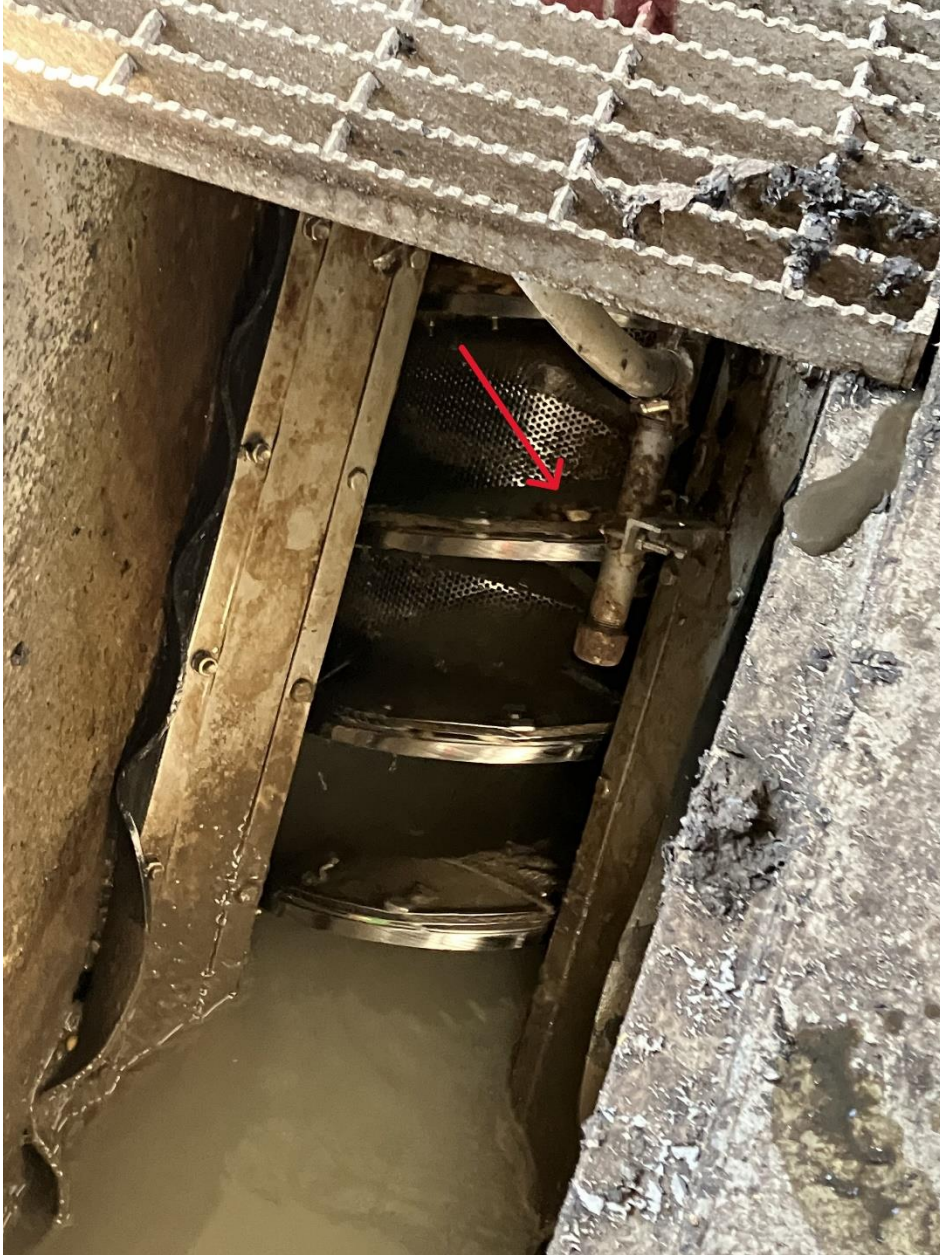
1- Lakeside Fine Screen Auger with Residual Gravel Noted
