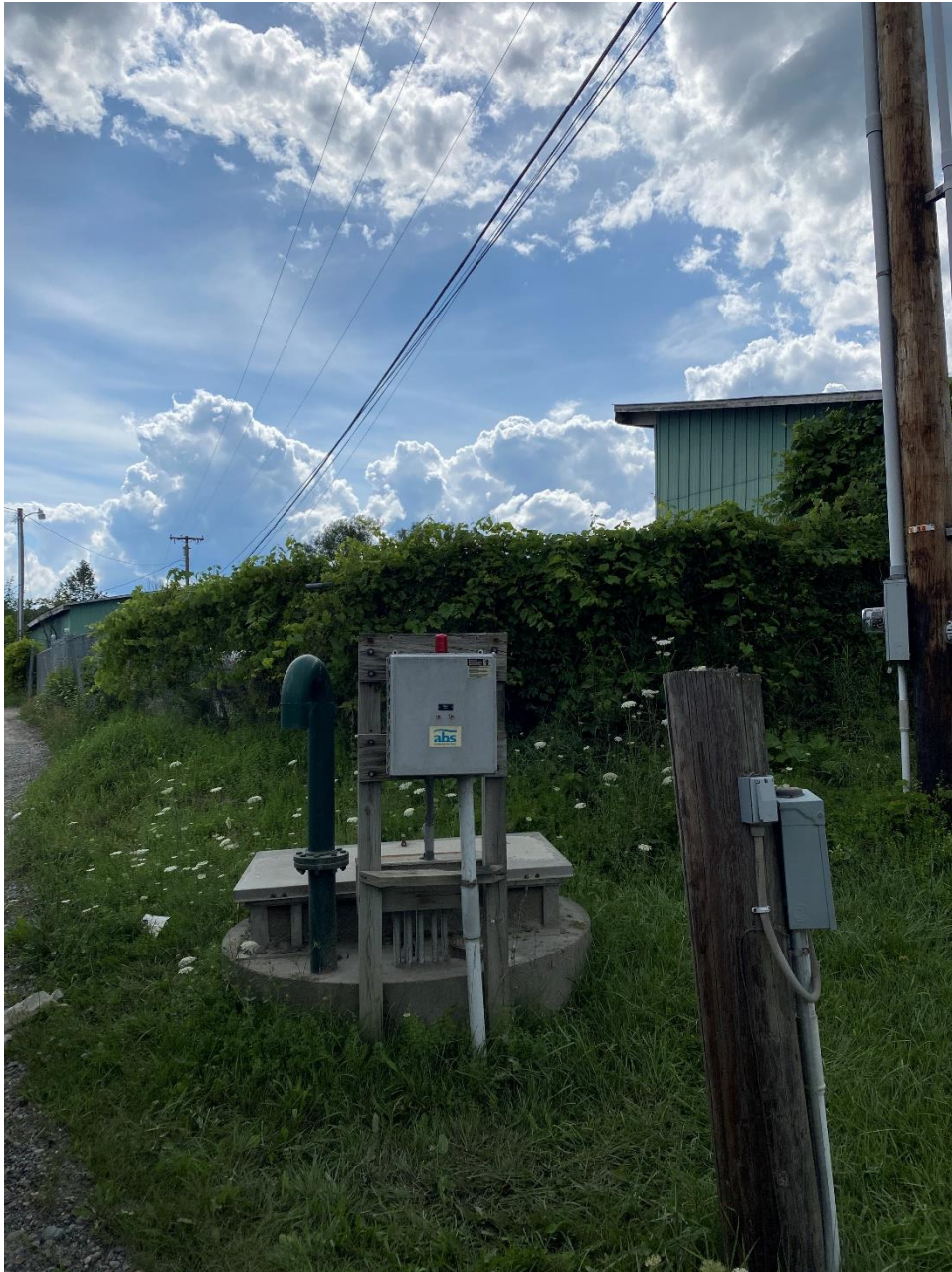
8- Blanchard Oil Pump Station with Control/Electrical Panel (Photo Courtesy of Chief Operator Phil Laramie)
