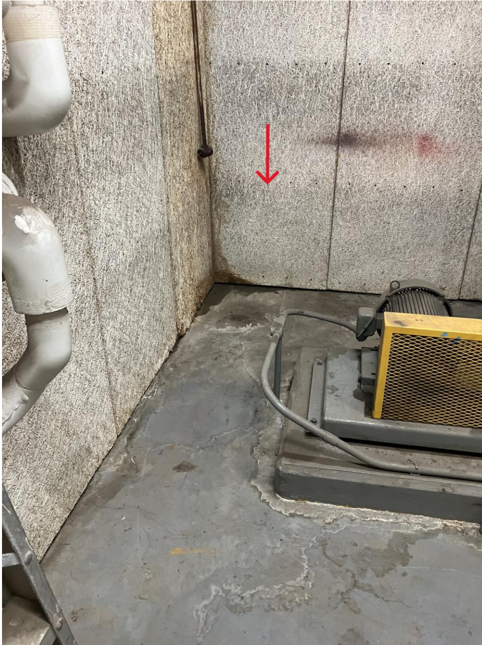
3- Blower Room Showing High Water Mark at Approximately 2 Feet
