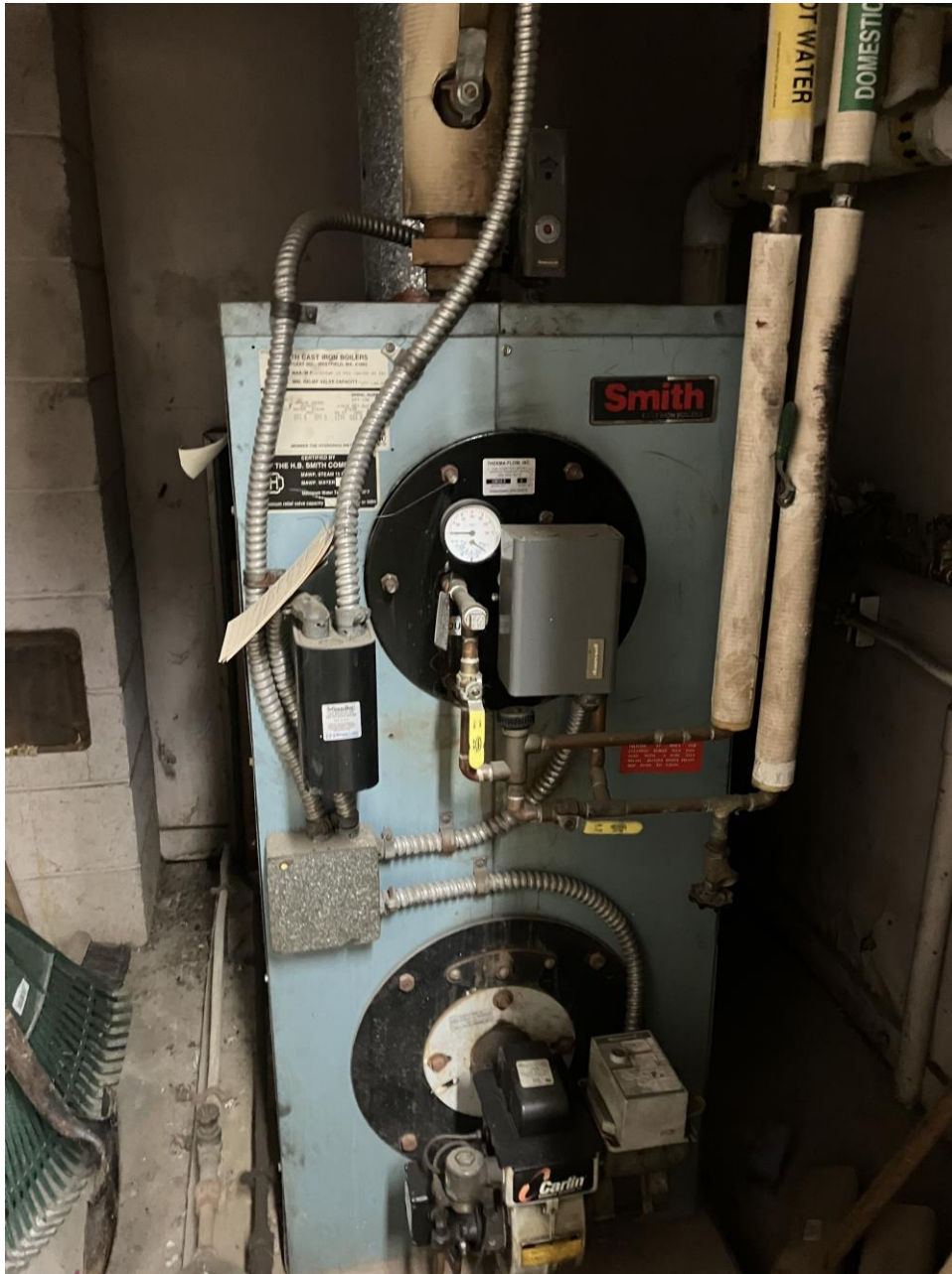
4- Smith Boiler in Basement of Main Building
