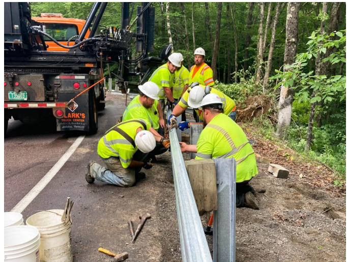
FAYSTON. Many maintenance projects require collaboration among different district garages, like this guardrail repair along VT Route 17 that saw three different crews team up to remove, replace, and clean up the project area in one efficient afternoon.
