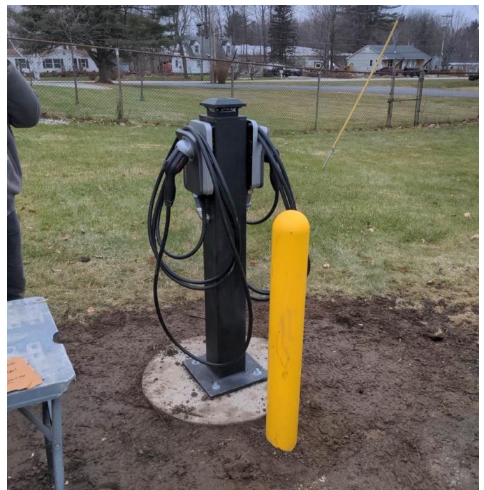
BENNINGTON. The Agency installed new Level 2 EV chargers at AOT Maintenance District garages throughout the state.
