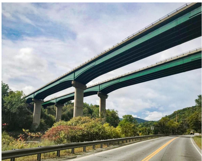
SHARON. Bridge repairs along I-89 over the White River in Sharon were completed this year. Work included rehabilitating both bridge decks with all structural steel stripped and recoated.
