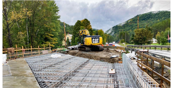
CHESTER. A multi-year bridge replacement project began along VT Route 103 in Spring 2022. The bridge deck has been replaced and minor repairs were made to the bridge piers, beams, and bearings. Crews will return in Spring 2023 to complete work on expansion joints, landscaping, and punch list items.
