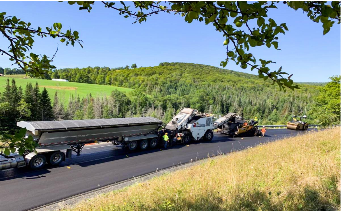
CHELSEA - THETFORD. In 2022, a 15-mile paving project on VT Route 113 was completed. The project included a full-depth reclamation of the roadway, superelevation correction, new guardrail, improved signage, drainage, and more.
