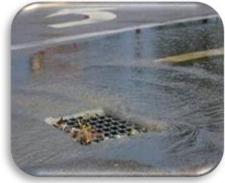
Photo: Road stormwater collection
