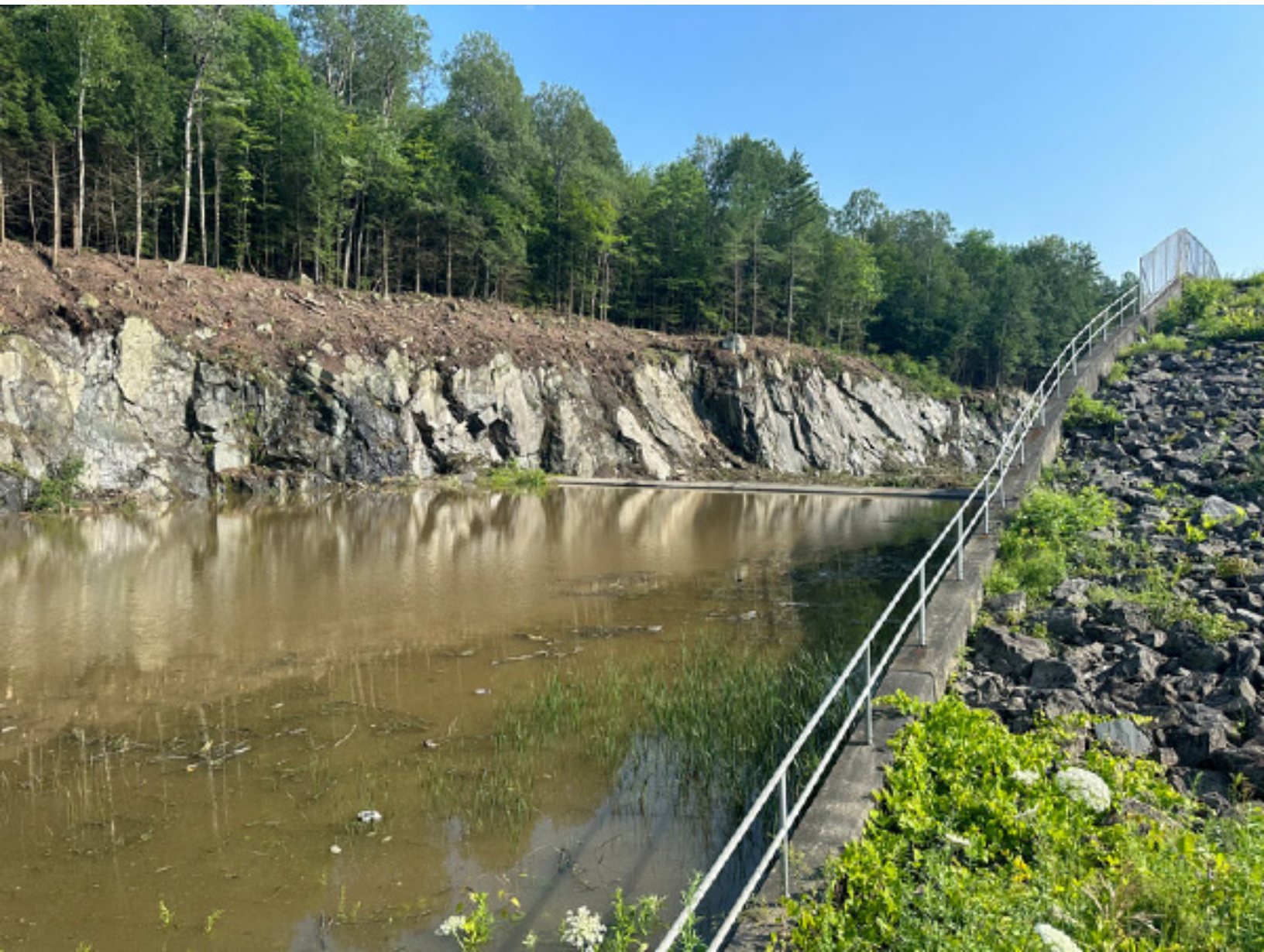
Wrightsville Dam following significant rainfall on July 12, 2023 Photo Credit: Wrightsville Beach Recreation District
