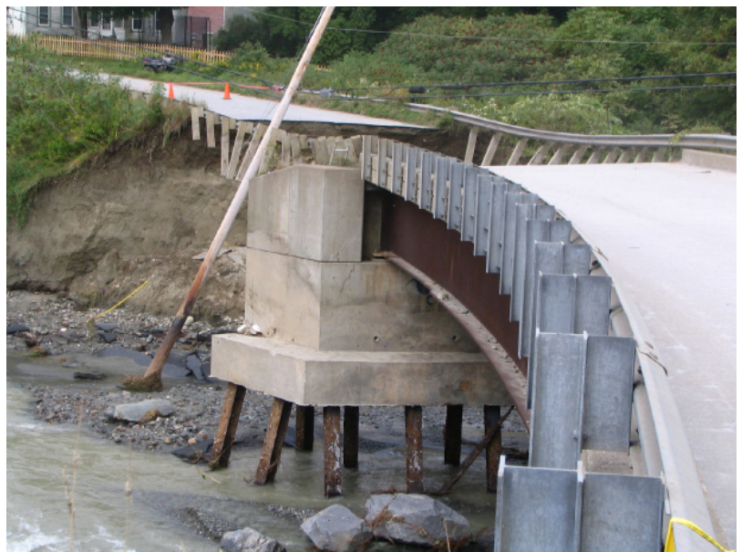
Significant scour along the Riford Brook in Braintree caused severe damage to Riford Brook Road during Tropical Storm Irene.
