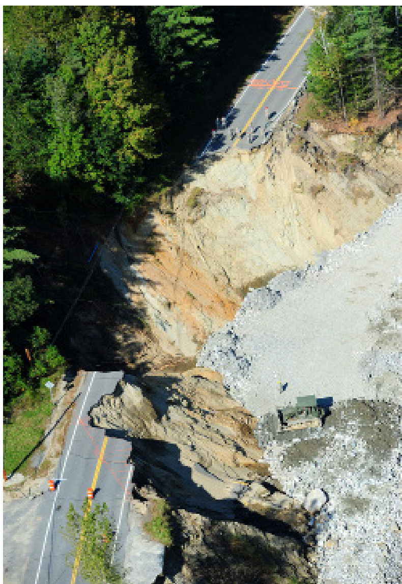
Route 131 in Cavendish devastated by slope failure. Photo Credit: www.mansfieldheliflight.com/flood/
