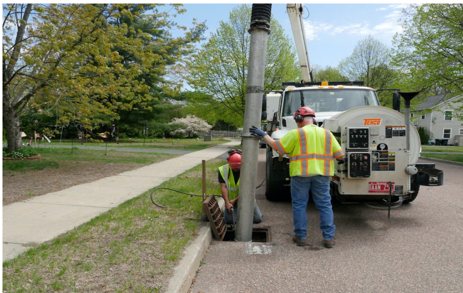
Members of the City of South Burlington stormwater maintenance crew clean a catch basin with a Vactor 2100 jet/vac Truck.
