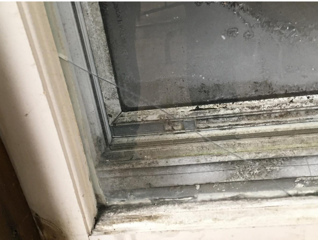
Suspicious looking mold and cracked glass at Arvin A Brown Library, Richford, VT.
