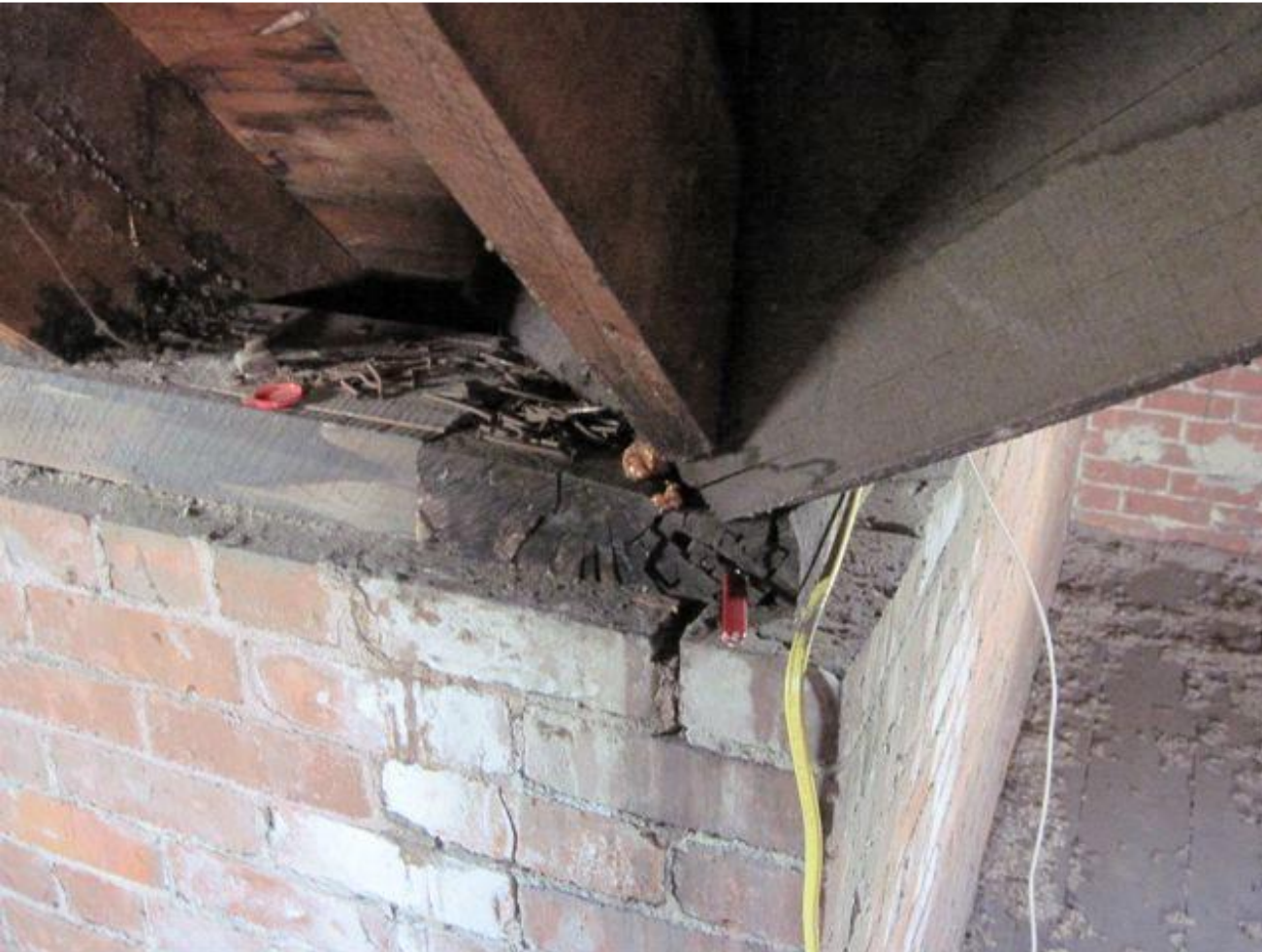
Critical structural rot and pedestal damage supporting the roof at the Weathersfield Proctor Library, Weathersfield, VT
