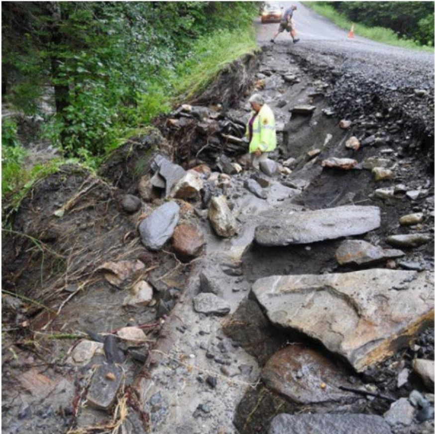
Storm damage assessment in Cabot
